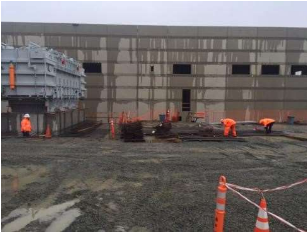
Figure 3 – APEC installed rebar at the transformer pad. View south, January 22, 2016. Photo courtesy of PG&E.
