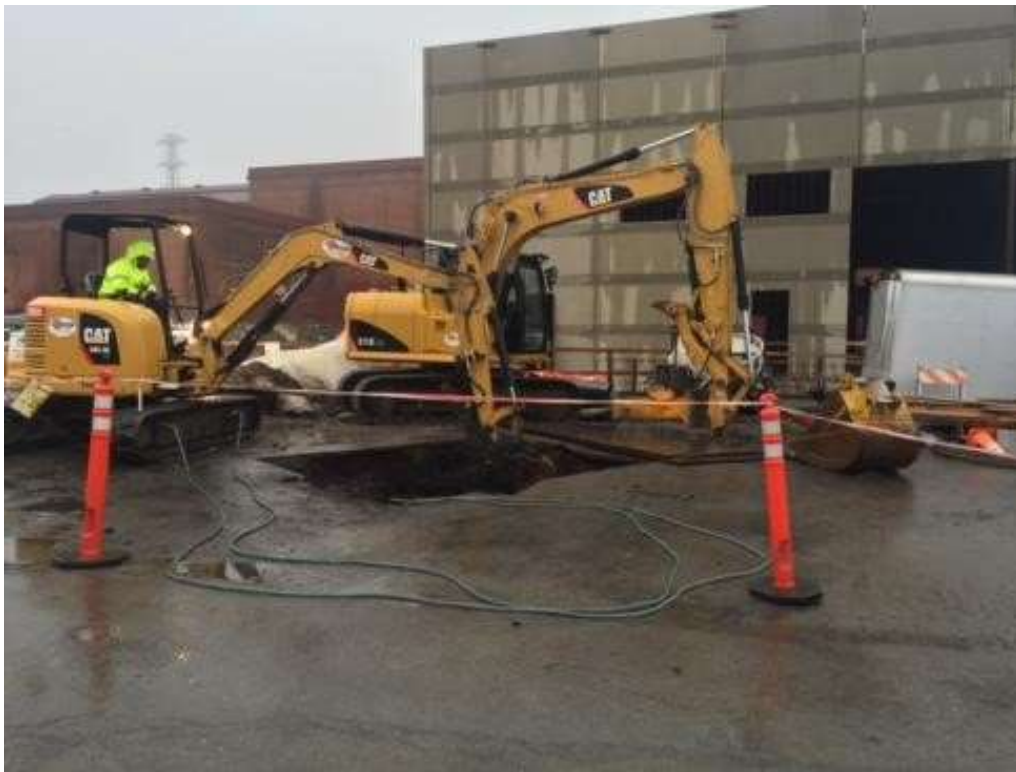
Figure 2 – APEC excavated a concrete footing west of the GIS building. View east, January 22, 2016. Photo courtesy of PG&E.
