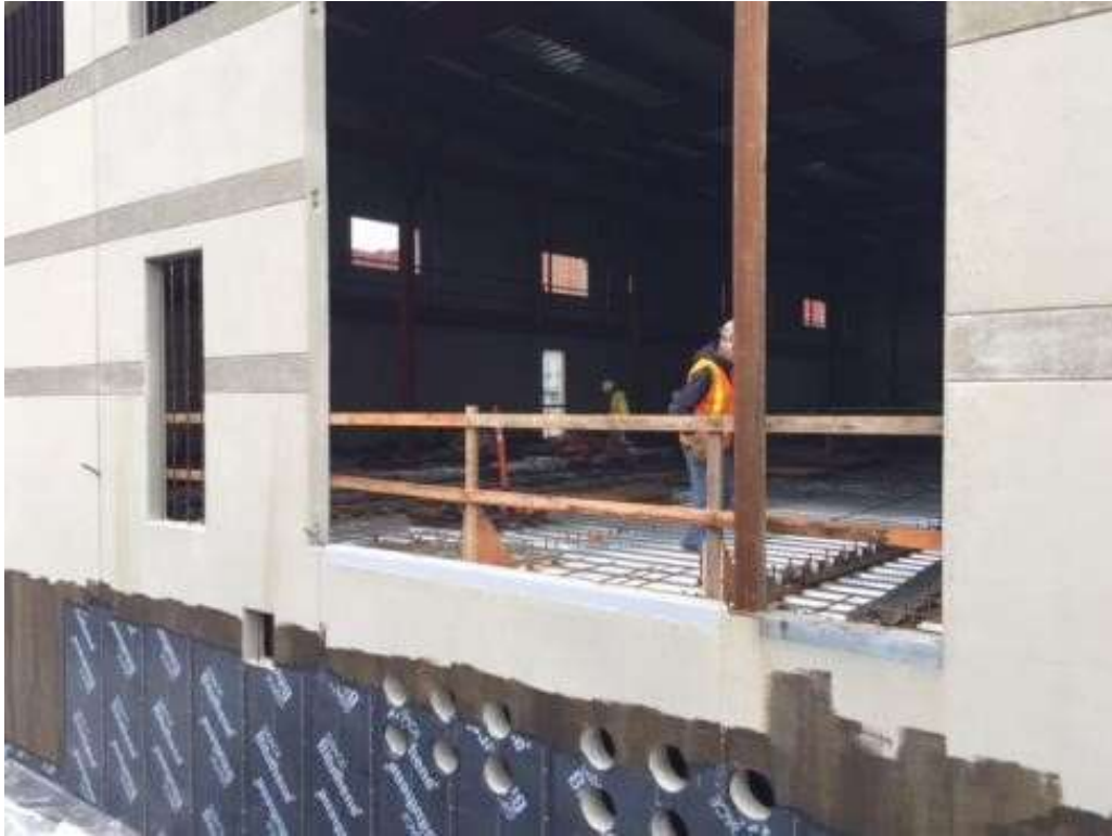
Figure 1 – B.T. Mancini installed studs on the pan decking in GIS building. View northeast, January 20, 2016. Photo courtesy of PG&E.
