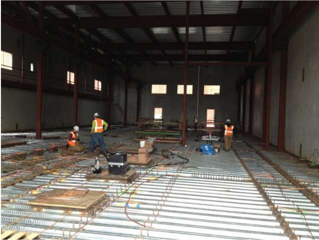
Figure 1 – Crews welding and conducting electrical work in the GIS building. View east, January 28, 2016.
