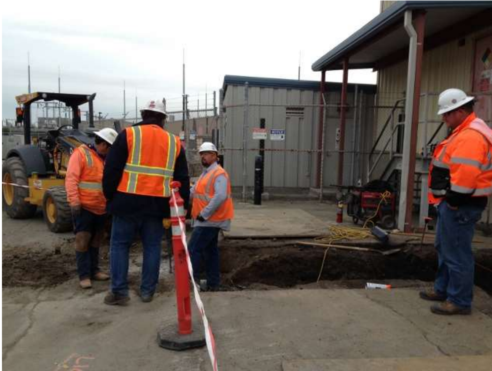
Figure 3 – Crews excavating a trench for GIS building power cable. View south, January 28, 2016.
