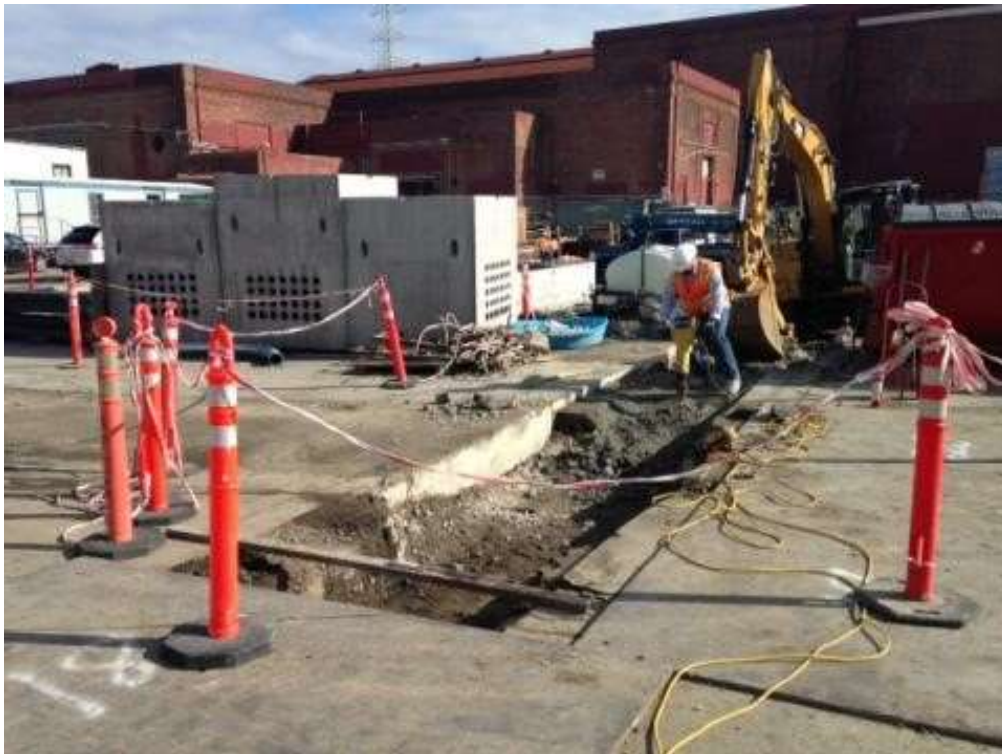
Figure 2 – APEC excavating for cable trench. View east, February 3, 2016. Photo courtesy of PG&E.
