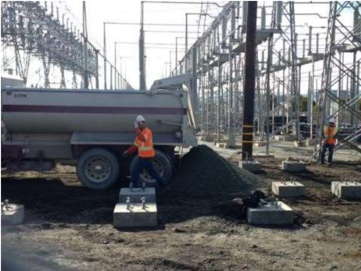
Figure 5 – APEC backfilled trenches and laid out baserock in adjacent substation. View south, February 3, 2016. Photo courtesy of PG&E.
