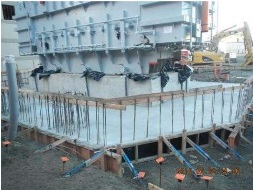
Figure 4 – APEC poured concrete at the transformer pad. View southwest, February 5, 2016. Photo courtesy of PG&E.
