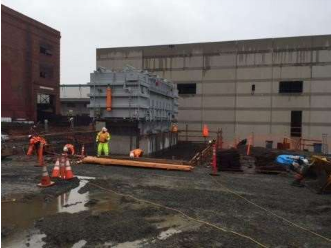
Figure 3 – APEC built concrete forms at the transformer pad. View south, February 2, 2016. Photo courtesy of PG&E.
