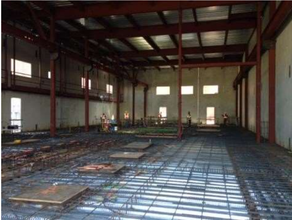
Figure 1 – Crews working in the GIS building. View east, February 3, 2016. Photo courtesy of PG&E.
