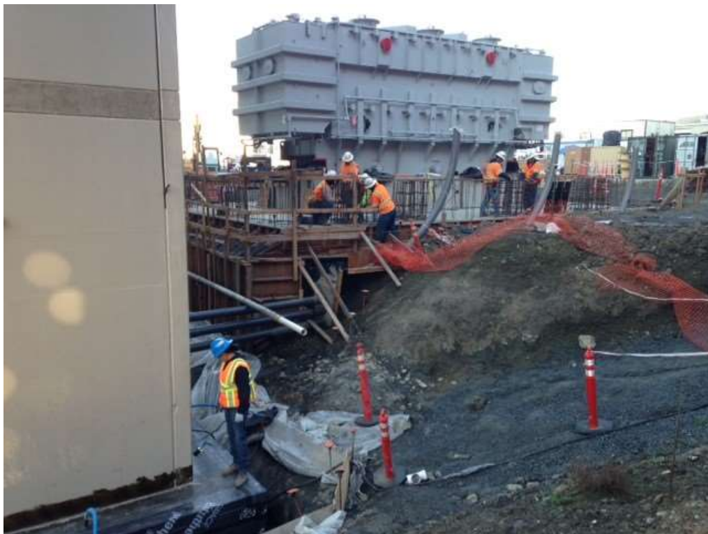
Figure 2 – APEC installing forms at transformer pad and ERS waterproofing GIS building. View northwest, February 9, 2016. Photo courtesy of PG&E.
