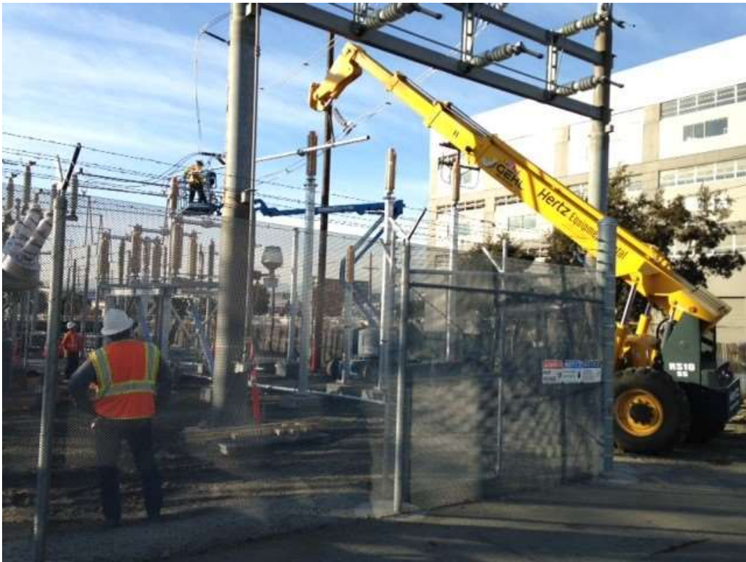
Figure 3 – CCE installing infrastructure in substation. View northwest, February 9, 2016. Photo courtesy of PG&E.
