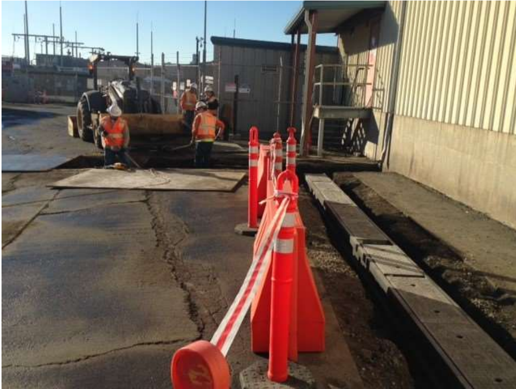
Figure 1 – APEC excavating for cable trench in Switchyard. View south, February 8, 2016. Photo courtesy of PG&E.
