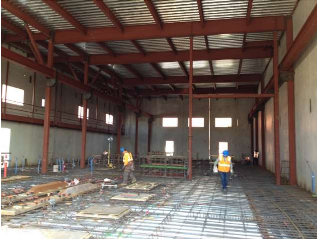
Figure 1 – Crews preparing for concrete pour on first floor of the GIS building. View east, February 24, 2016.
