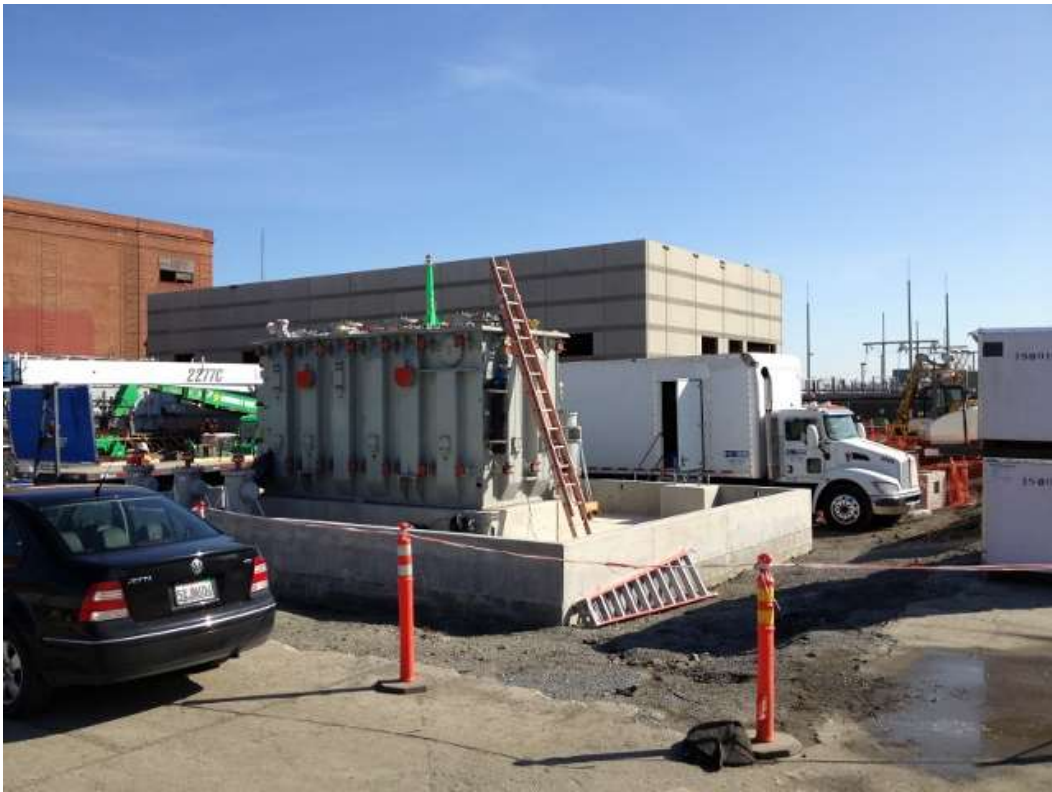
Figure 3 – Crews installing radiators, adding oil, and testing the reactor. View southeast, February 24, 2016.
