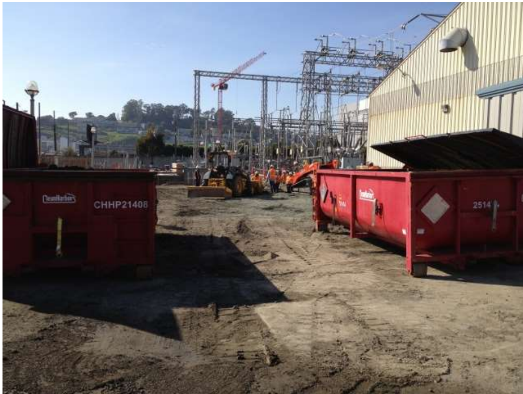
Figure 4 – Crews were excavating in the substation for the 115 kV line. View west, February 24, 2016.
