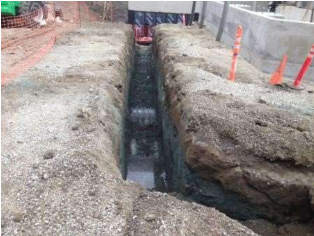
Figure 3 – Crews excavated near the transformer pad. View east, March 3, 2016. Photo courtesy of PG&E.
