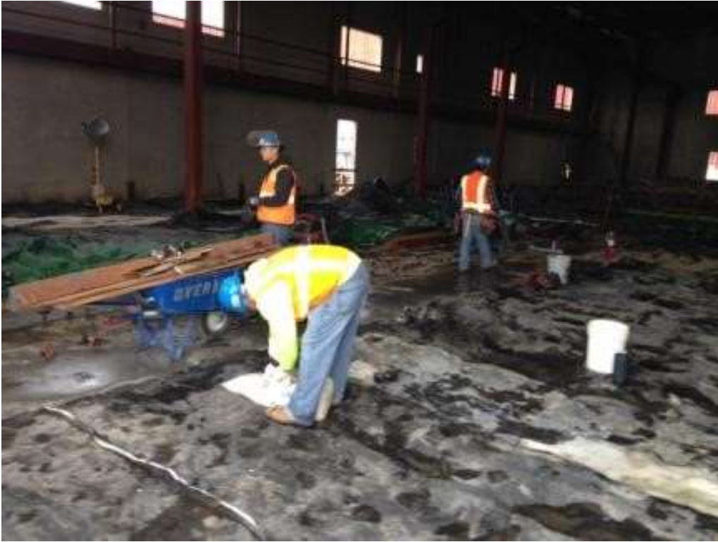
Figure 1 – Crews adjusted concrete curing blankets in the GIS building. View northeast, February 29, 2016. Photo courtesy of PG&E.
