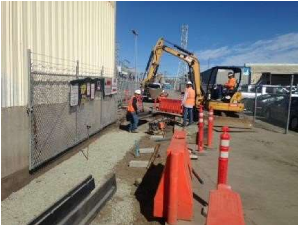
Figure 2 – Crews installing cable trays for the cable trench. View north, March 1, 2016. Photo courtesy of PG&E.
