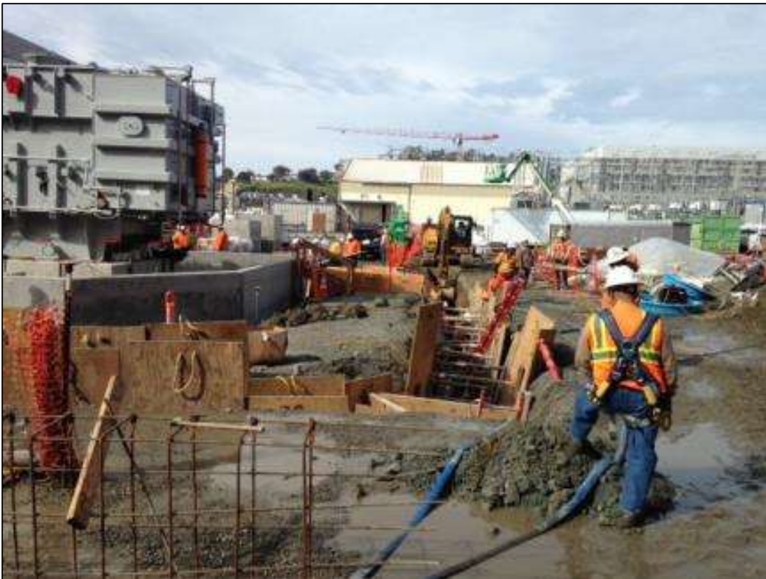
Figure 5 – Conditions at the switchyard site were very muddy during the subject reporting period given the recent rains. Photo courtesy of PG&E.
