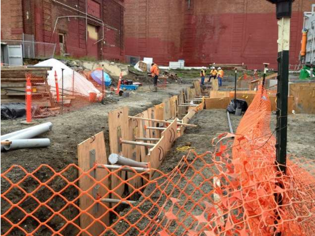
Figure 2 – Crews installing conduit in the trench line near the transformer. View east, March 9, 2016.
