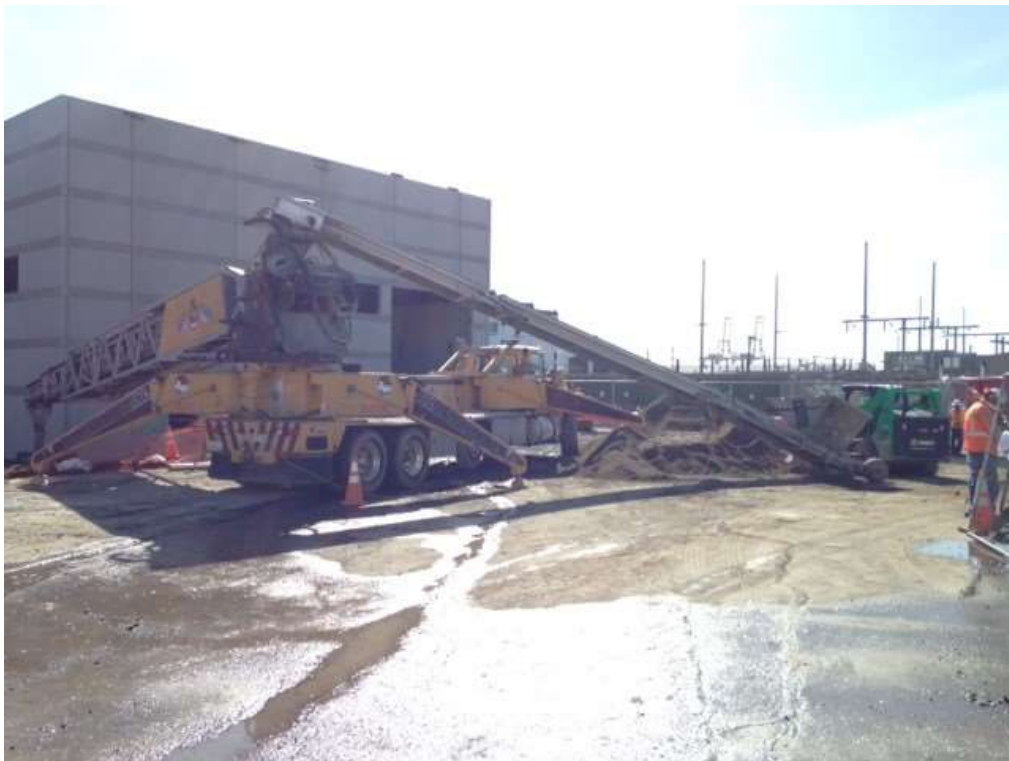
Figure 2 – Backfilling with baserock around the foundation of the GIS building. View southeast, March 15, 2016. Photo courtesy of PG&E.
