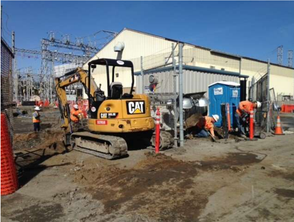
Figure 1 – APEC excavating the cable trench. View northwest, March 15, 2016. Photo courtesy of PG&E.
