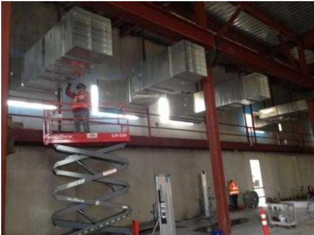
Figure 4 – CER installing infrastructure in the GIS building at the Potrero Switchyard. View northeast, March 23, 2016. Photo courtesy of PG&E.
