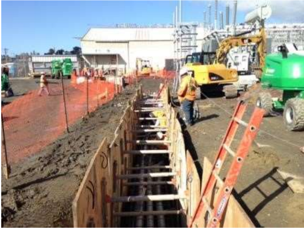
Figure 1 – APEC installing conduit in duct bank trench in the Potrero Switchyard. View west, March 22, 2016. Photo courtesy of PG&E.
