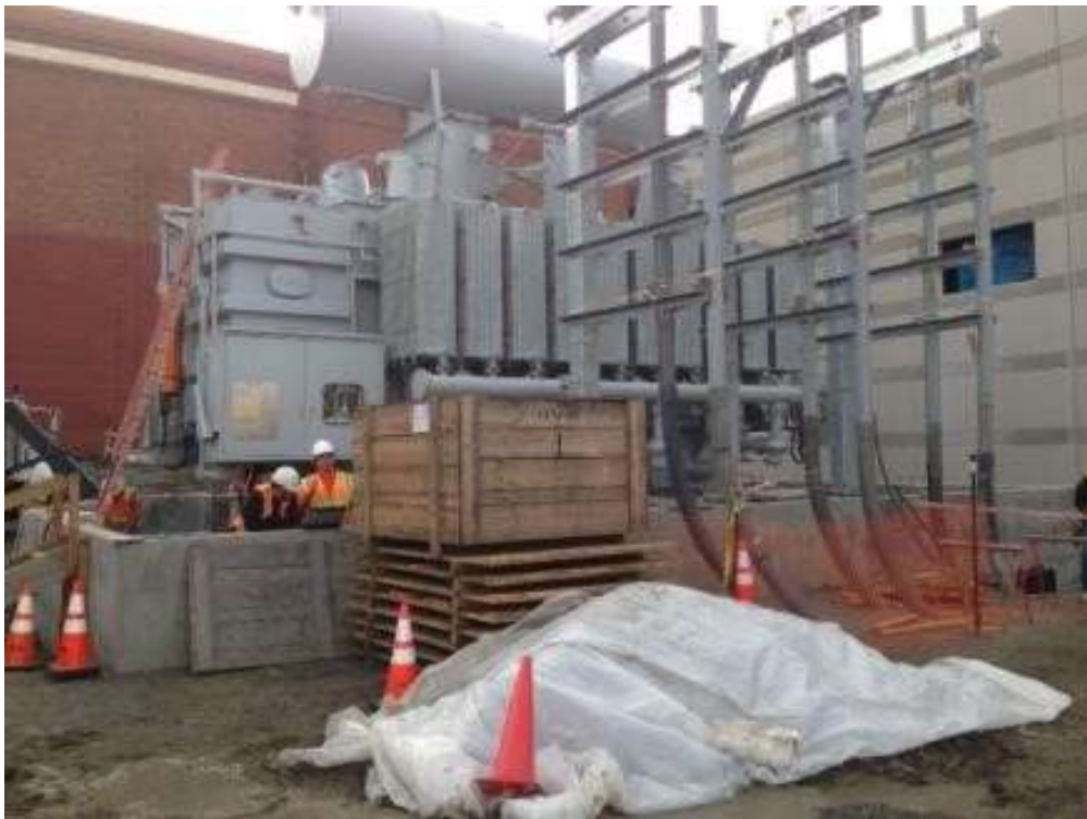
Figure 2 – NASS assembling the transformer in the Potrero Switchyard. View east, March 23, 2016. Photo courtesy of PG&E.
