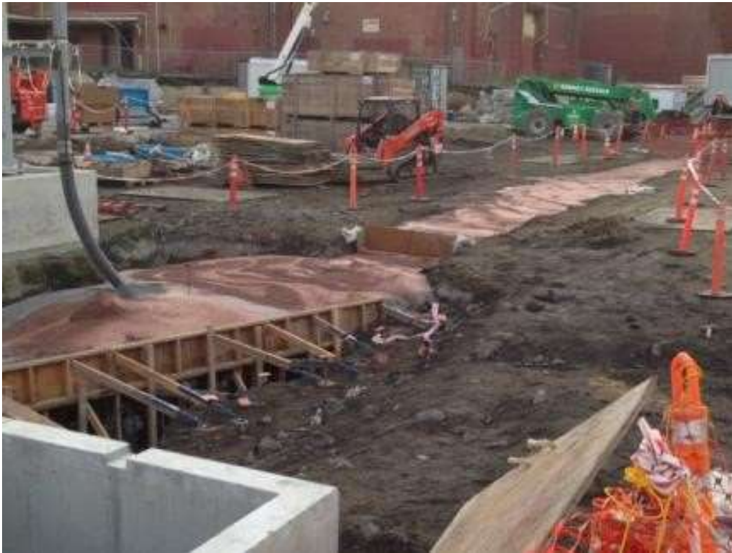
Figure 3 – Proven backfilling duct bank trench with cement slurry in the Potrero Switchyard. View east, March 23, 2016. Photo courtesy of PG&E.
