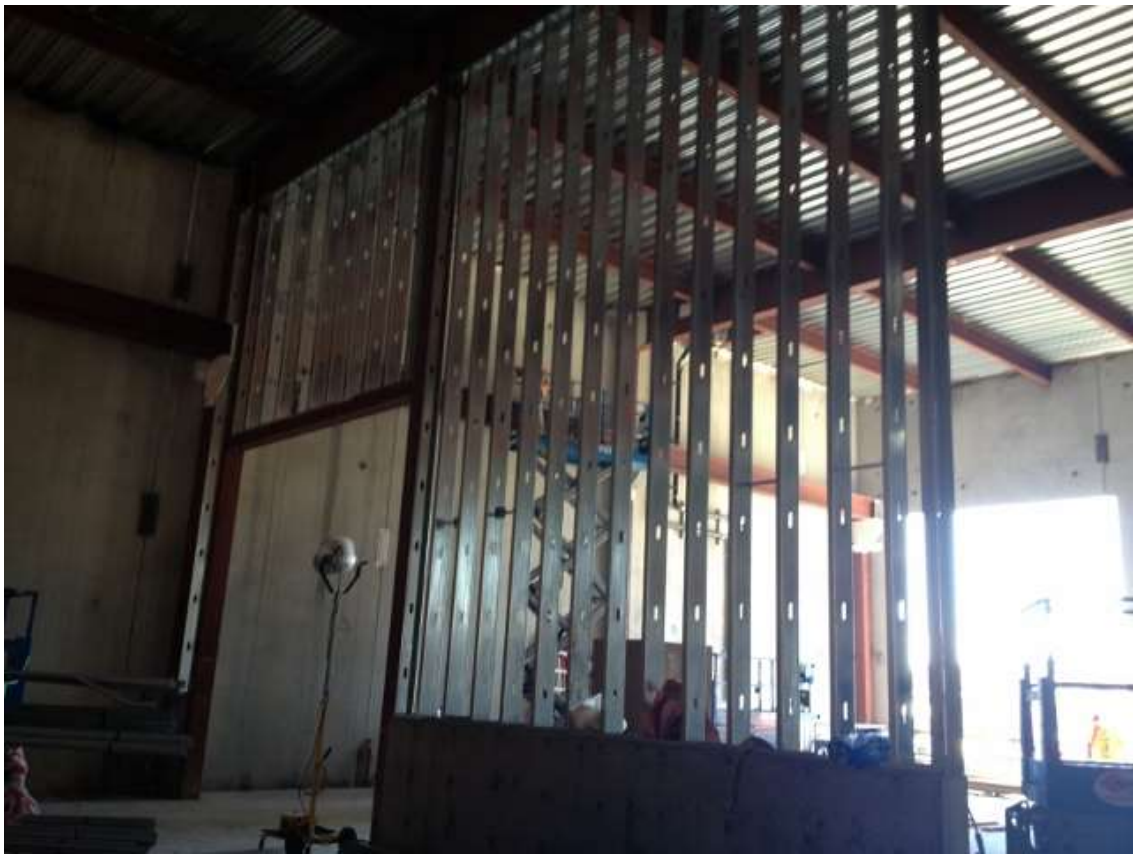
Figure 5 – Bayside conducted framing work in the GIS building at the Potrero Switchyard. View southwest, March 31, 2016.
