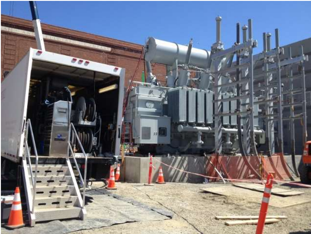
Figure 3 – Crews working on assembling the transformer in the Potrero Switchyard. View east, March 31, 2016.
