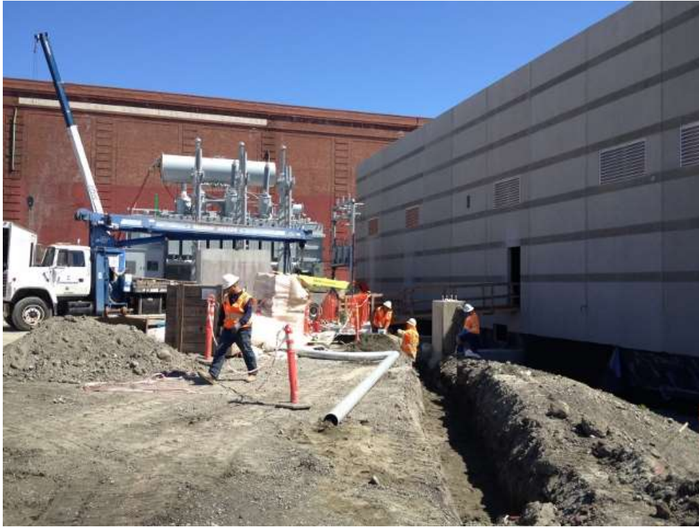
Figure 1 – APEC excavating trench and installing cable trays and cable in the Potrero Switchyard. View east, March 31, 2016.
