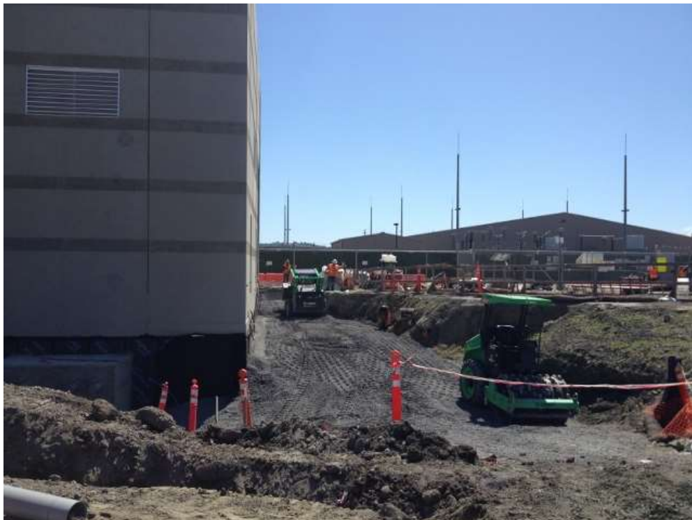
Figure 2 – Proven distributed and compacted baserock around the foundation of the GIS building. View south, March 31, 2016.
