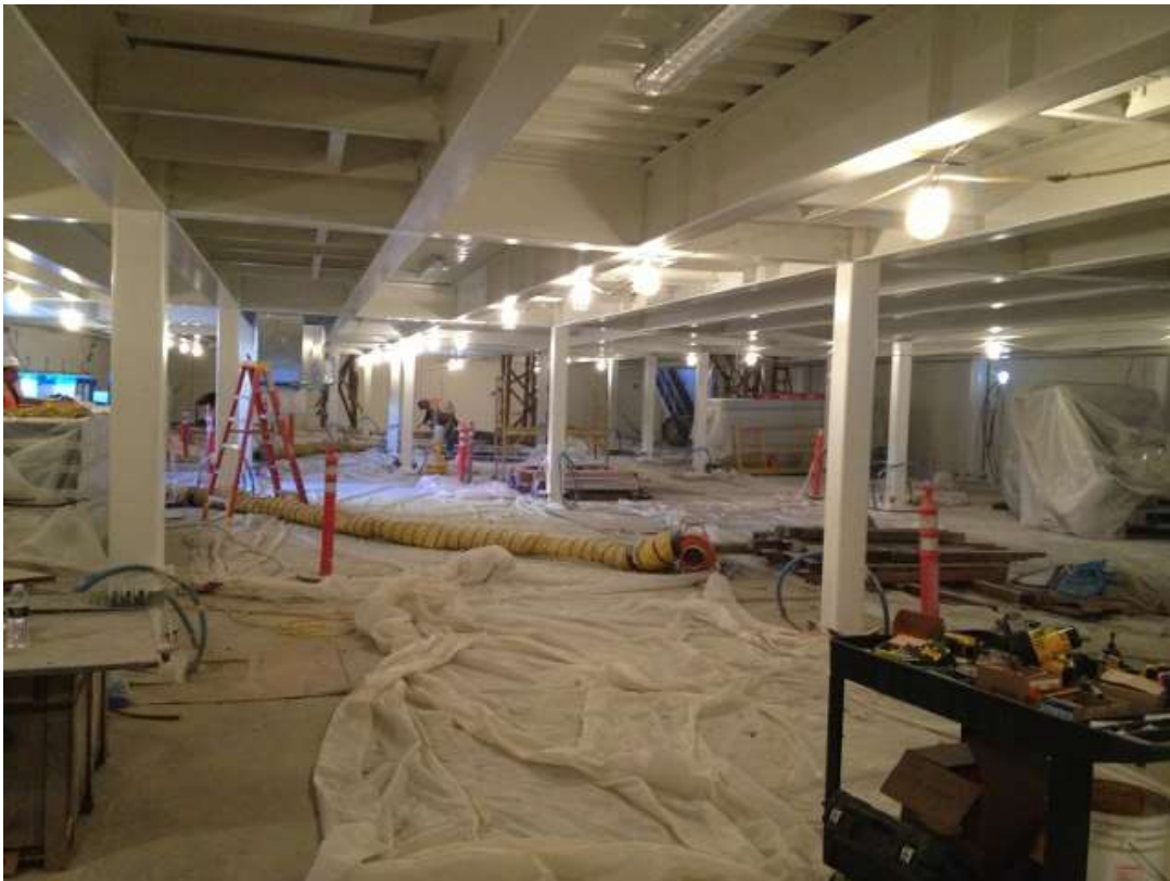
Figure 4 – VPI painted in the GIS building at the Potrero Switchyard. View east, March 31, 2016.
