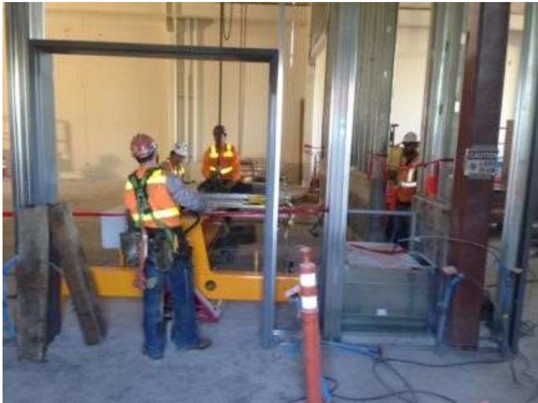
Figure 4 – Bayside conducted framing work in the GIS building at the Potrero Switchyard. View south, April 6, 2016. Photo courtesy of PG&E.
