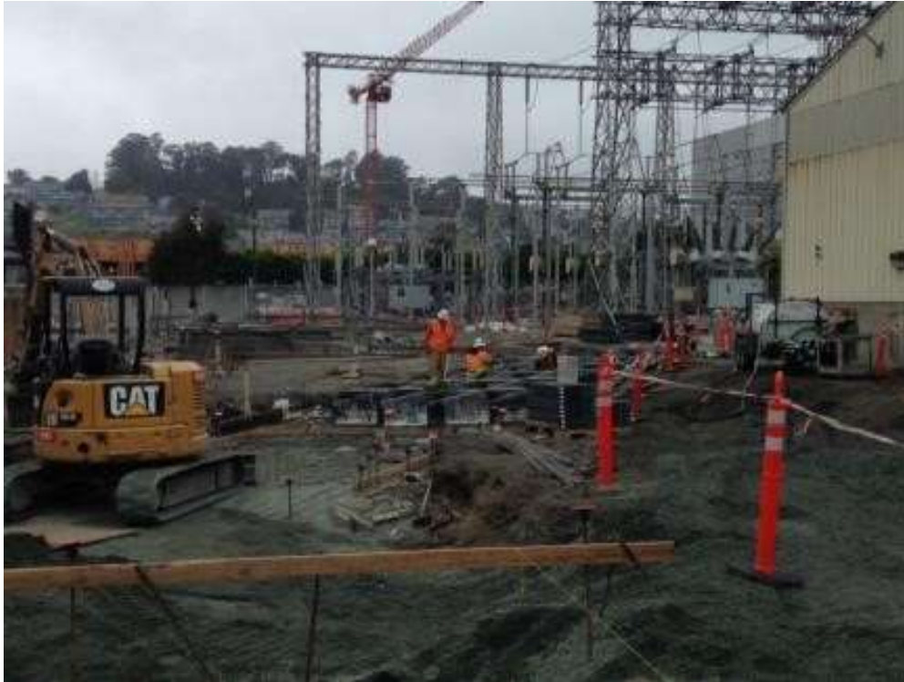
Figure 1 – APEC installing cable trays in the trench in the Potrero Switchyard. View west, April 8, 2016. Photo courtesy of PG&E.
