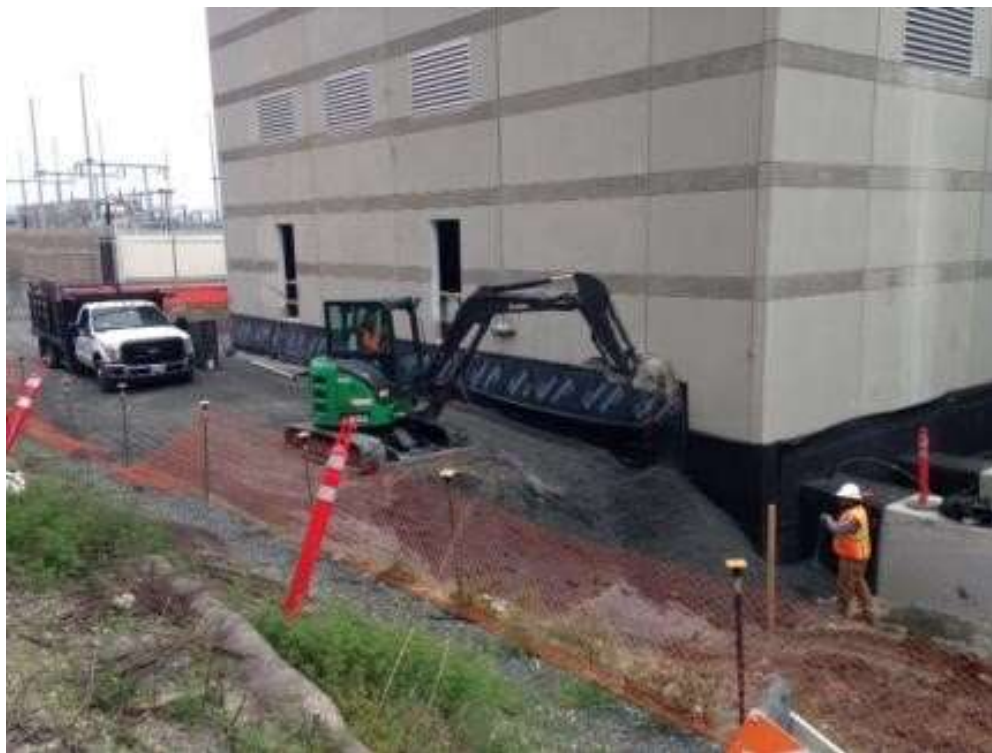
Figure 2 – Proven distributed and compacted baserock around the foundation of the GIS building at the Potrero Switchyard. View southwest, April 8, 2016. Photo courtesy of PG&E.
