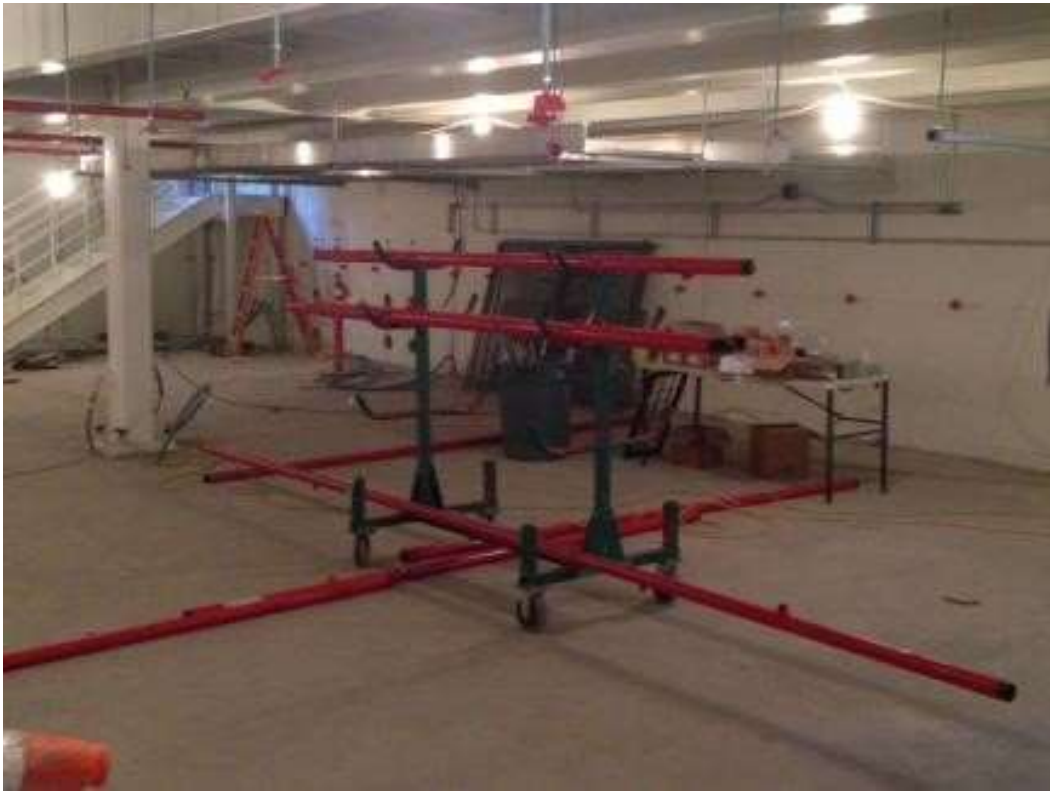
Figure 3 – Cosco installed sprinklers in the GIS building basement at the Potrero Switchyard. View northwest, April 7, 2016. Photo courtesy of PG&E.
