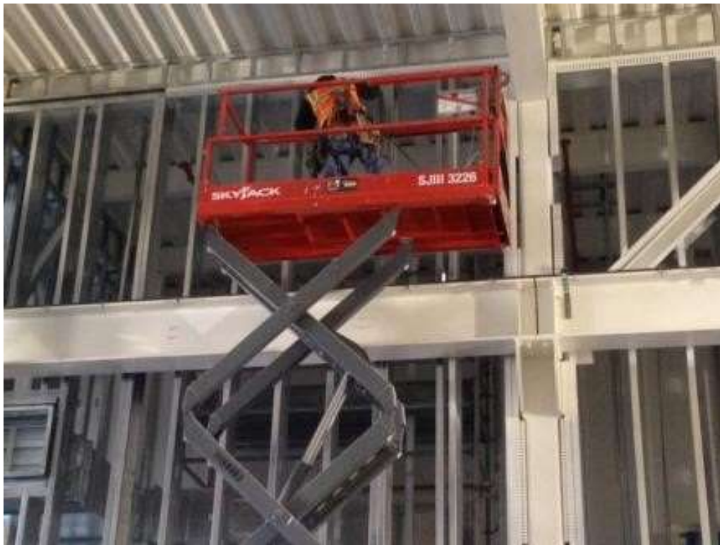
Figure 2 – Bayside conducted framing work in the GIS building at the Potrero Switchyard. View east, April 14, 2016. Photo courtesy of PG&E.
