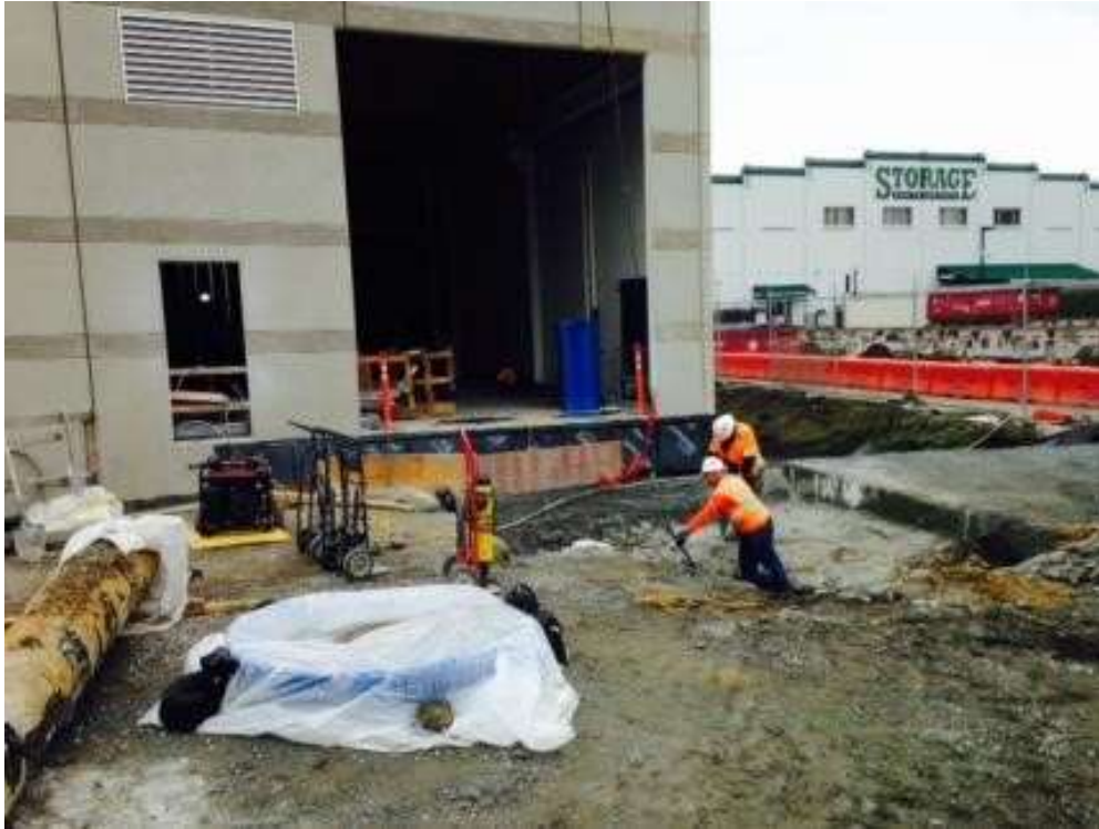
Figure 1 – APEC jackhammered concrete and excavated west of the GIS building. View southeast, April 11, 2016. Photo courtesy of PG&E.
