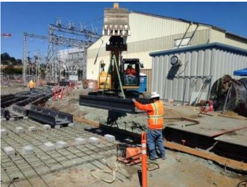
Figure 4 – APEC installing cable trays in the trench at the substation. View northwest, April 15, 2016. Photo courtesy of PG&E.
