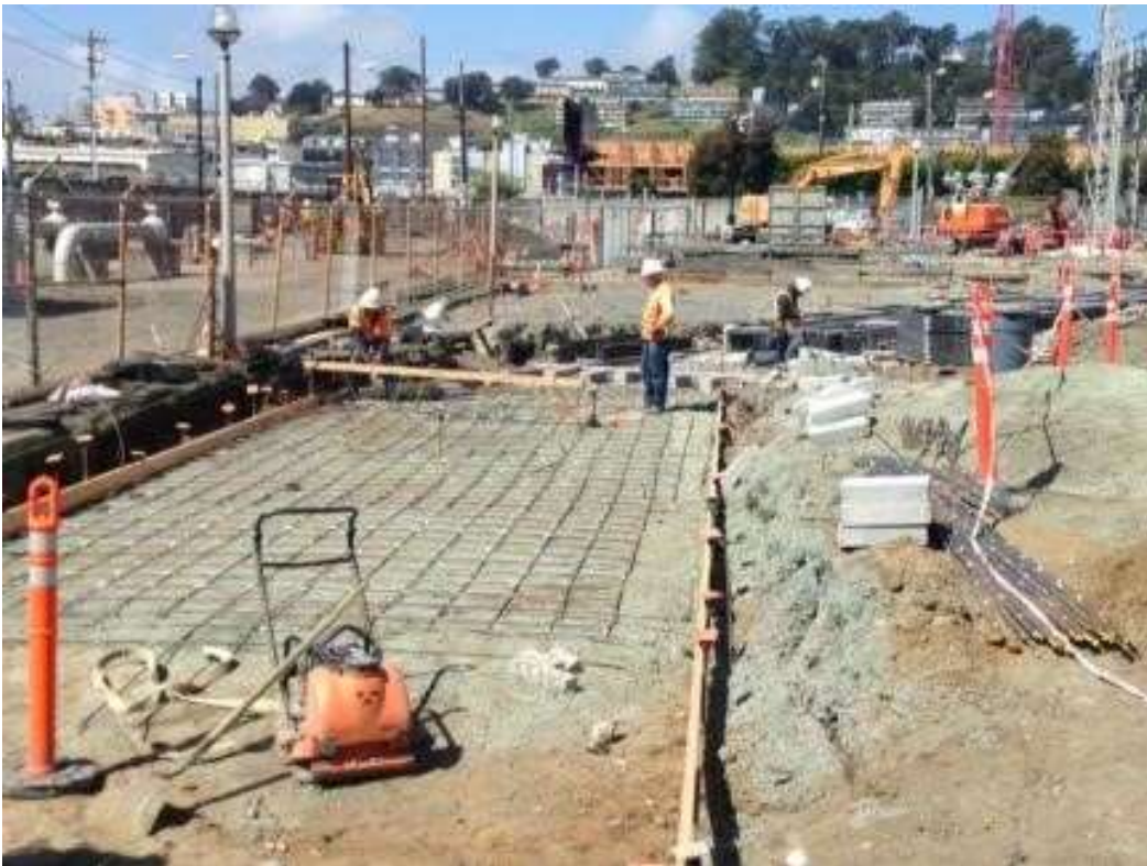
Figure 3 – APEC installing rebar in the trenches in the substation. View west, April 13, 2016. Photo courtesy of PG&E.
