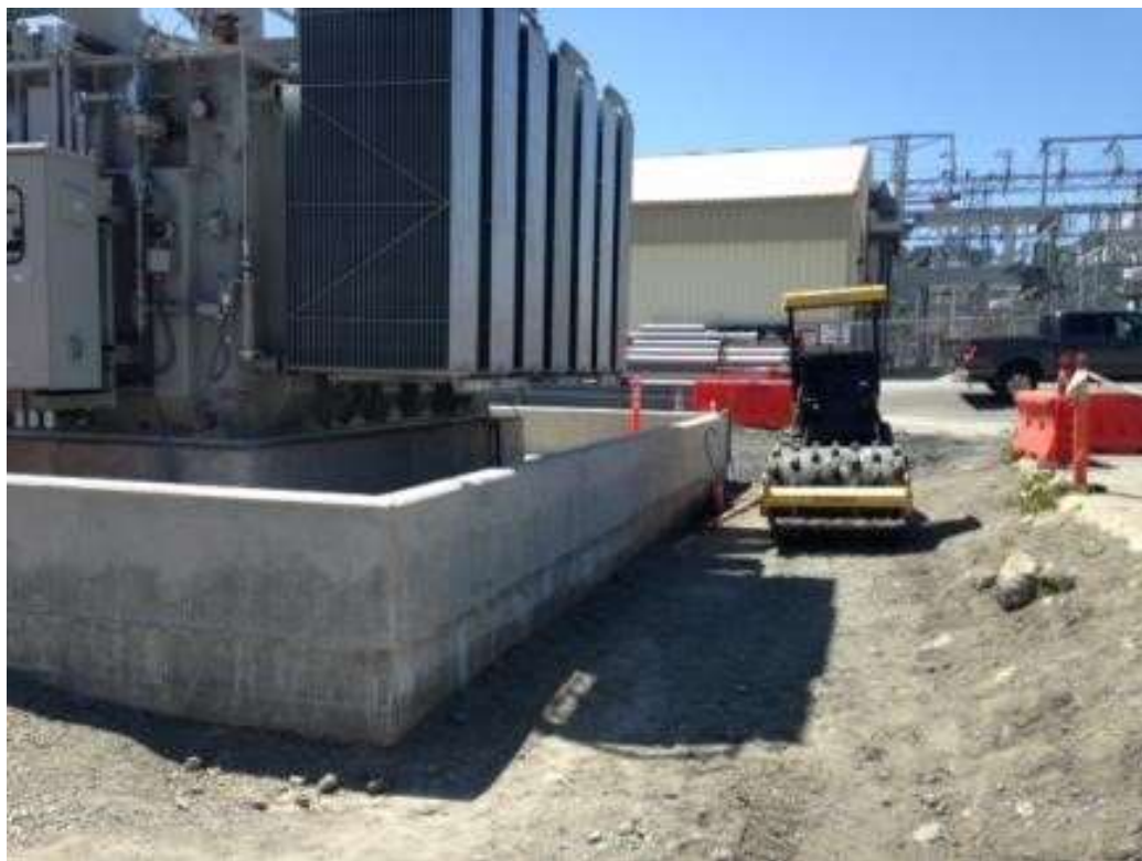
Figure 2 – APEC compacting backfill around reactor pad in the Potrero Switchyard. View west, April 25, 2016. Photo courtesy of PG&E.
