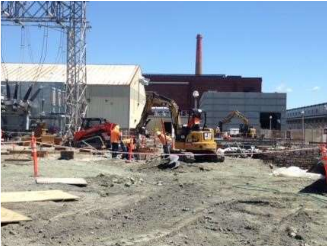
Figure 4 – APEC excavating trench in the substation. View east, April 25, 2016. Photo courtesy of PG&E.
