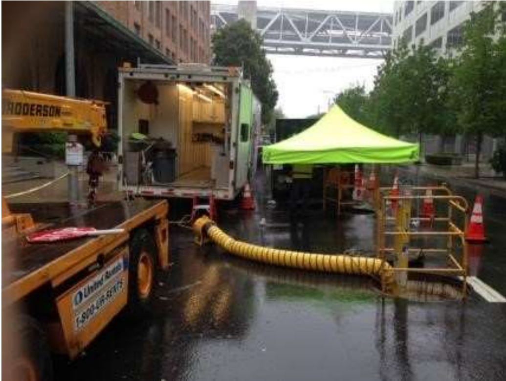
Figure 1 – Sumitomo conducting racking in transition vault on Spear St. View east, April 27, 2016. Photo courtesy of PG&E.
