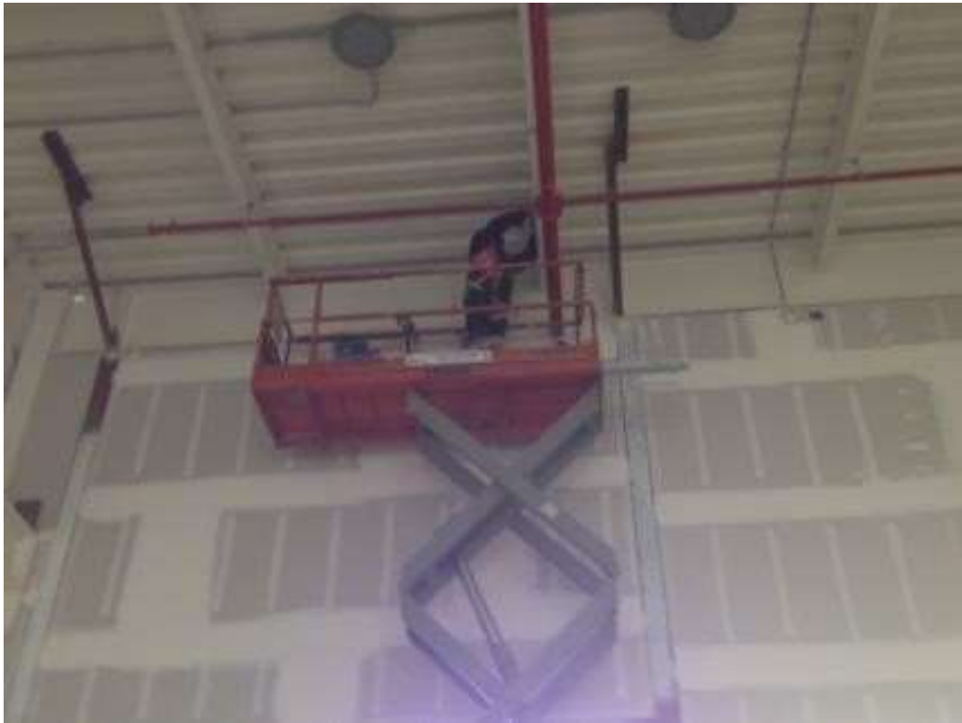
Figure 3 – Cosco installing sprinklers in the GIS building. View south, May 4, 2016. Photo courtesy of PG&E.
