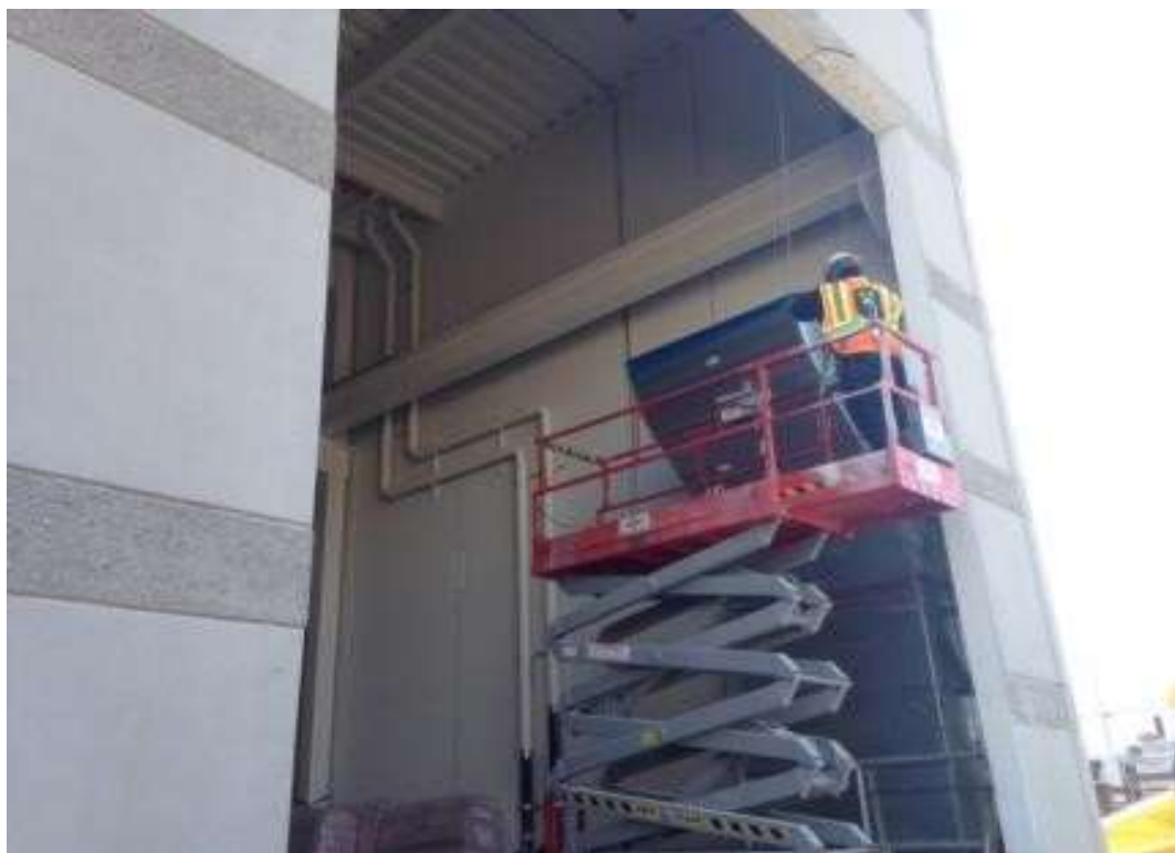
Figure 2 – CER installed infrastructure inside the GIS building. View southeast, May 2, 2016. Photo courtesy of PG&E.
