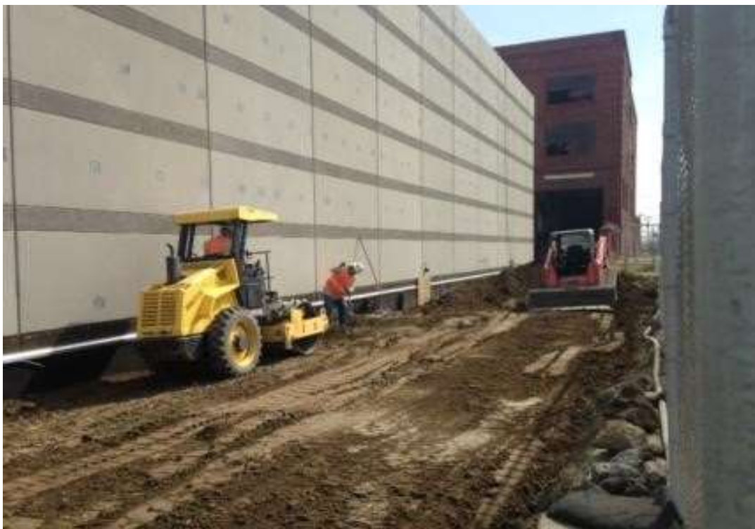
Figure 1 – APEC compacting backfill around the GIS building. View east, May 2, 2016. Photo courtesy of PG&E.
