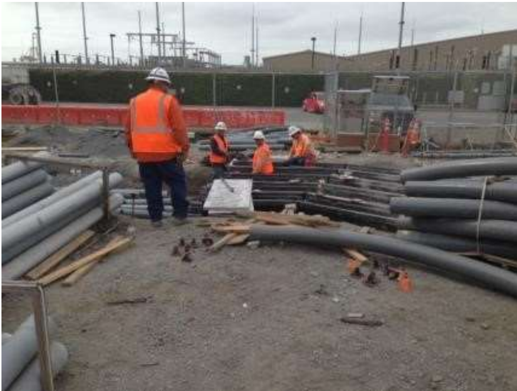
Figure 4 – APEC setting cable trench between GIS building and substation. View south, May 4, 2016. Photo courtesy of PG&E.
