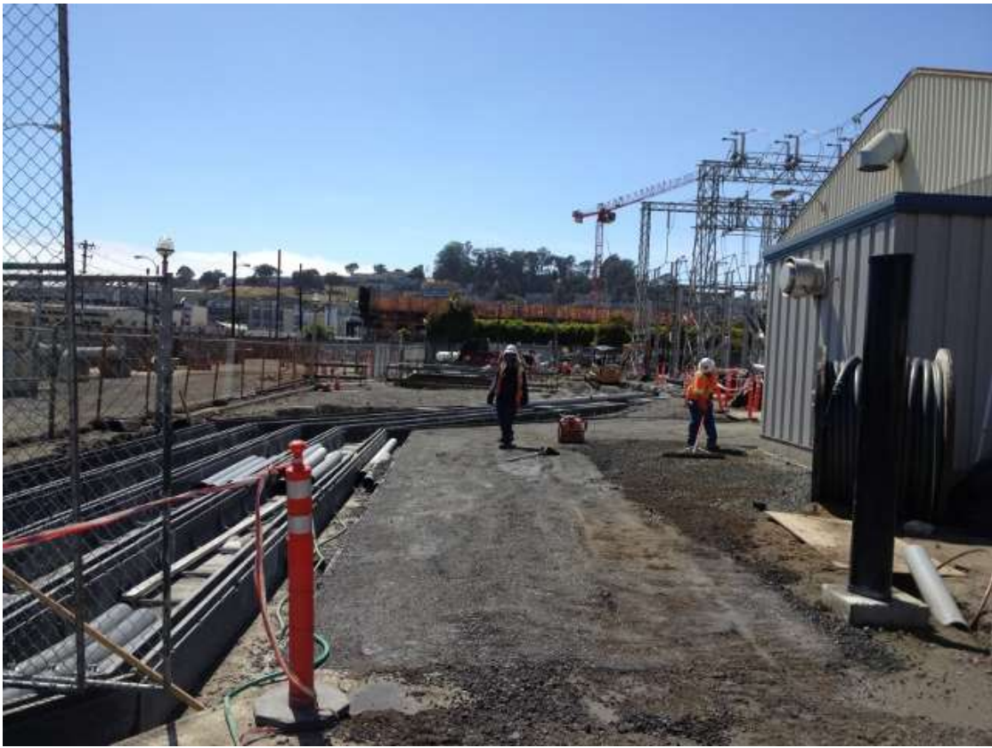
Figure 3 – Crews working on cable trench between GIS building and substation. View west, May 9, 2016.
