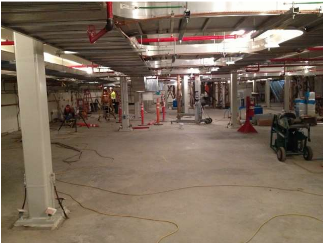
Figure 2 – CCE pulling wire in the GIS building from the reactor. View east, May 9, 2016.
