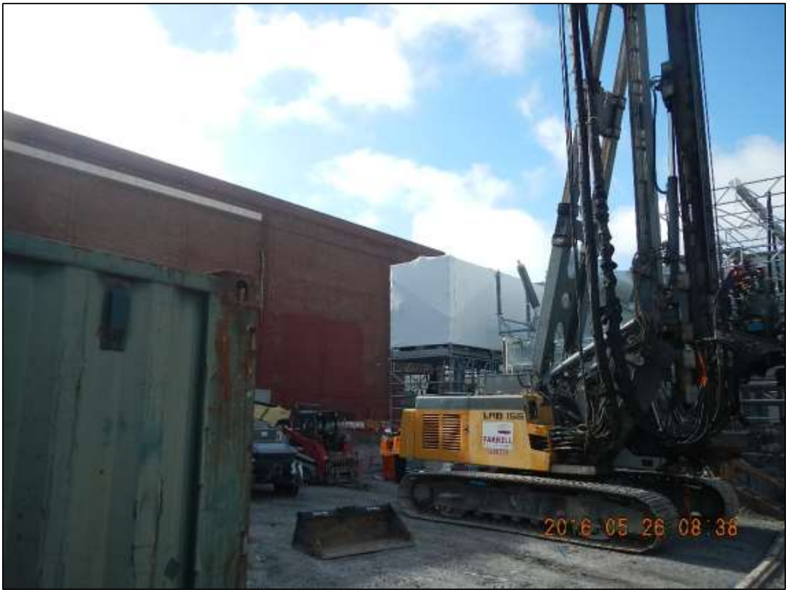
Figure 3: Farrell conducted drilling for a concrete block wall that will be going around the reactor/ transformer/ GIS building at Potrero Switchyard, May 26, 2016. Photo courtesy of PG&E.
