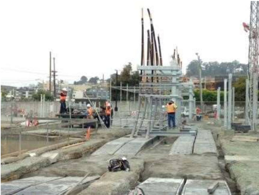
Figure 4: SSI installed scaffolding around the 115 kV bus in the substation, June 2, 2016. Photo courtesy of PG&E.
