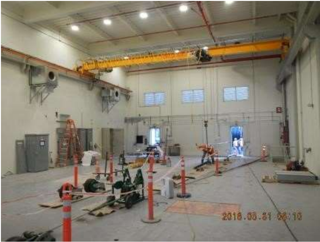
Figure 3: Metalset worked on the trolley beam in the GIS building, May 31, 2016. Photo courtesy of PG&E.
