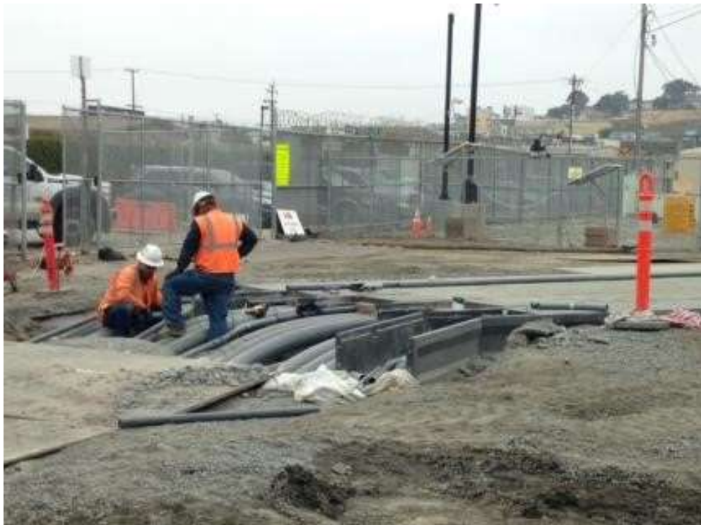
Figure 2: APEC installed conduit in the Potrero Switchyard, June 2, 2016. Photo courtesy of PG&E.
