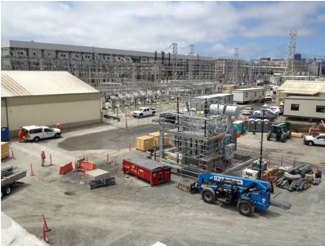
Figure 1: Overview of Potrero Switchyard from GIS rooftop, June 9, 2016.
