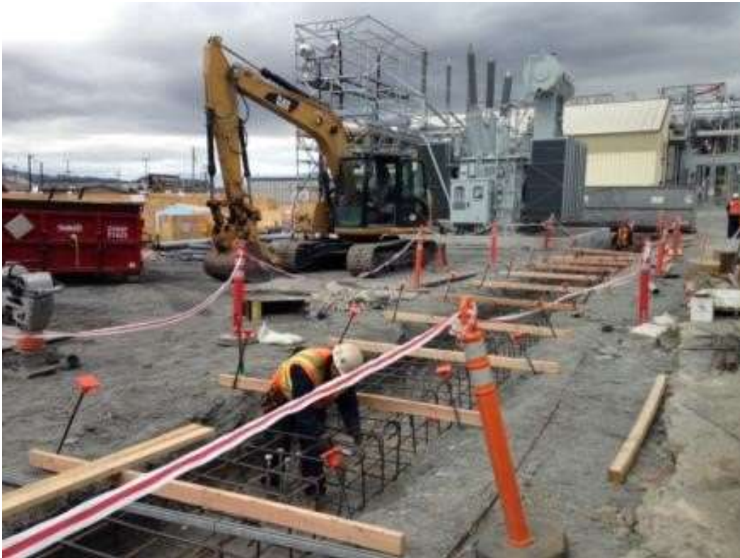
Figure 3: CMC installed rebar in the perimeter wall excavation, June 17, 2016. Photo courtesy of PG&E.
