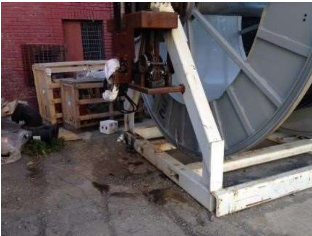
Figure 4: Secondary containment missing under cable reel machinery, June 14, 2016. Photo courtesy of PG&E.
