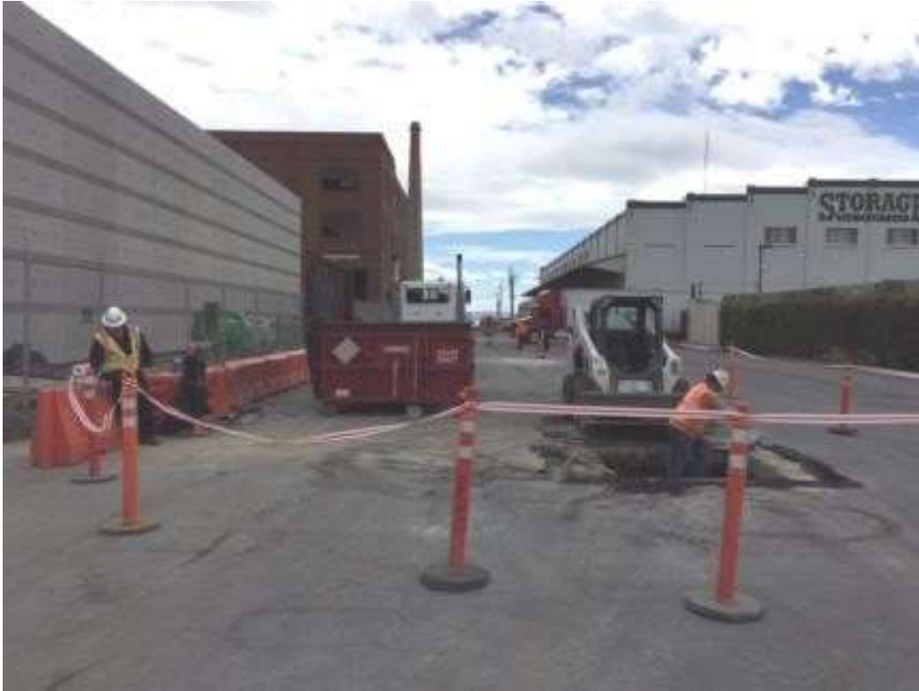
Figure 1: APEC excavating for the water and sewer line tie-in on 23 rd Street, June 17, 2016. Photo courtesy of PG&E.
