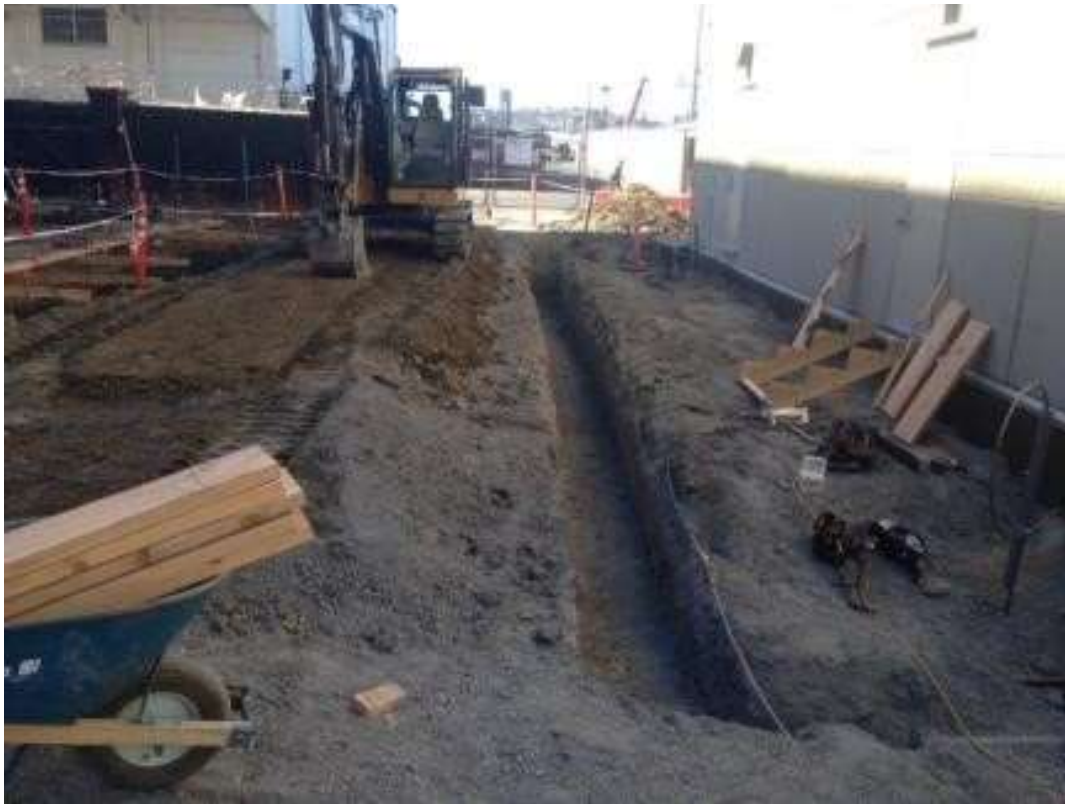
Figure 3: Proven excavated for the perimeter wall at the Potrero Switchyard, June 20, 2016. Photo courtesy of PG&E.
