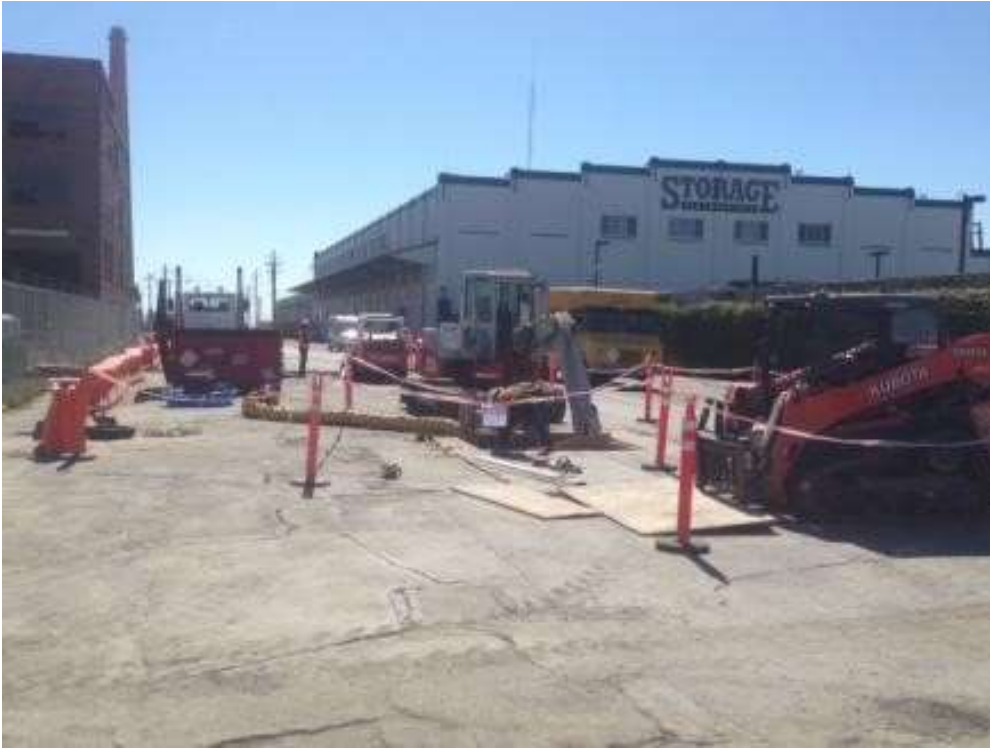
Figure 1: APEC excavating for the water and sewer line tie-in on 23 rd Street, June 23, 2016. Photo courtesy of PG&E.
