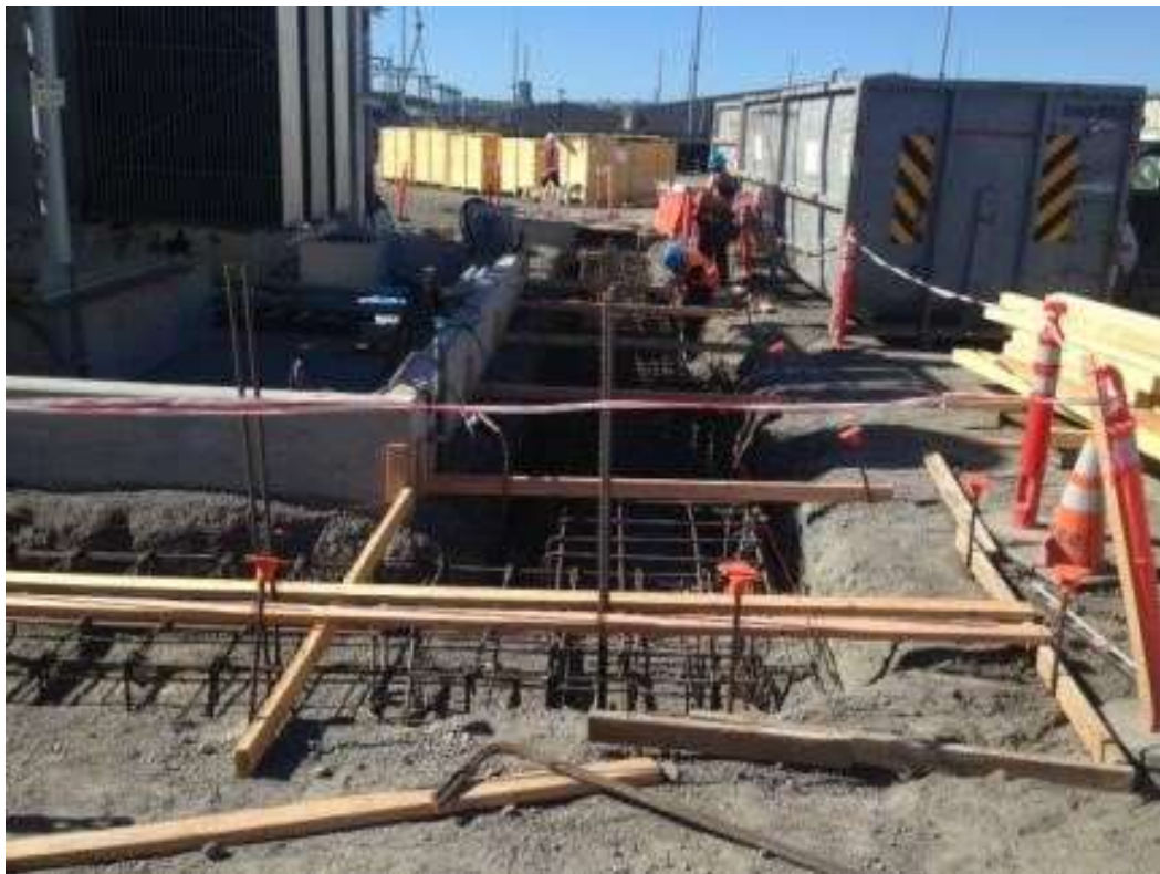
Figure 4: CMC installed rebar in perimeter wall footing at Potrero Switchyard, June 20, 2016. Photo courtesy of PG&E.
