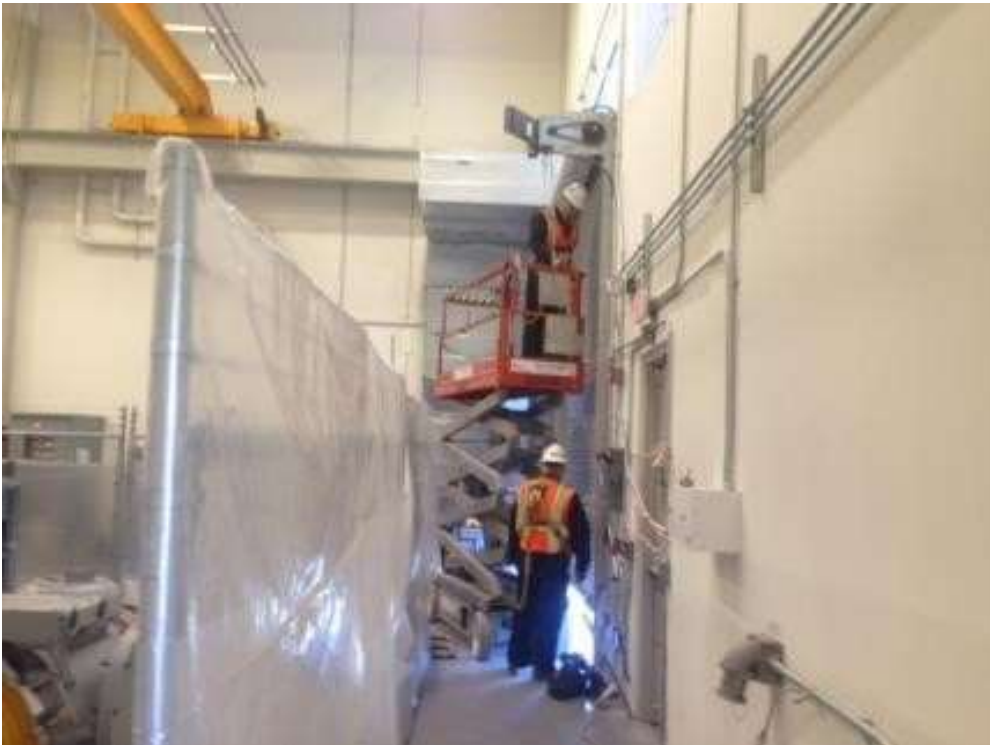
Figure 2: MEI conducting electrical work in GIS building, June 23, 2016. Photo courtesy of PG&E.
