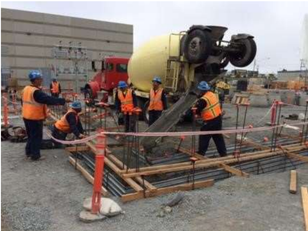
Figure 3: Overaa pouring concrete for perimeter wall at Potrero Switchyard, July 8, 2016. Photo courtesy of PG&E.
