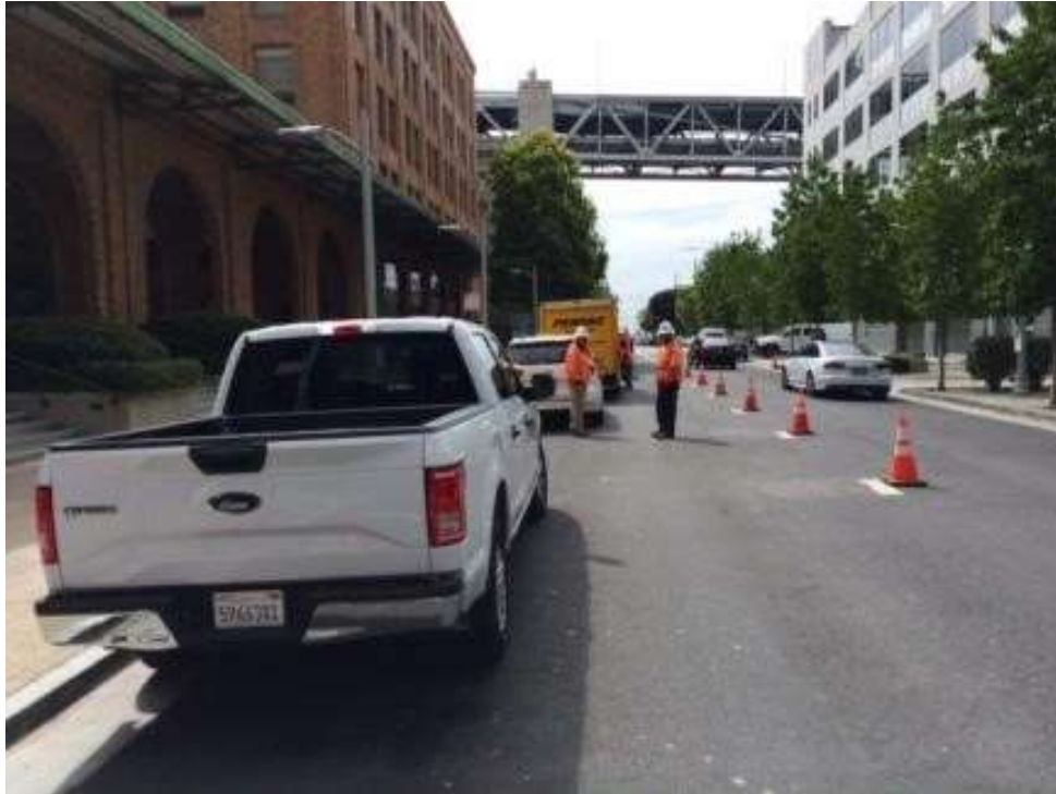
Figure 1: Sumitomo and NRE delivered equipment into the vault on Spear Street, July 8, 2016. Photo courtesy of PG&E.
