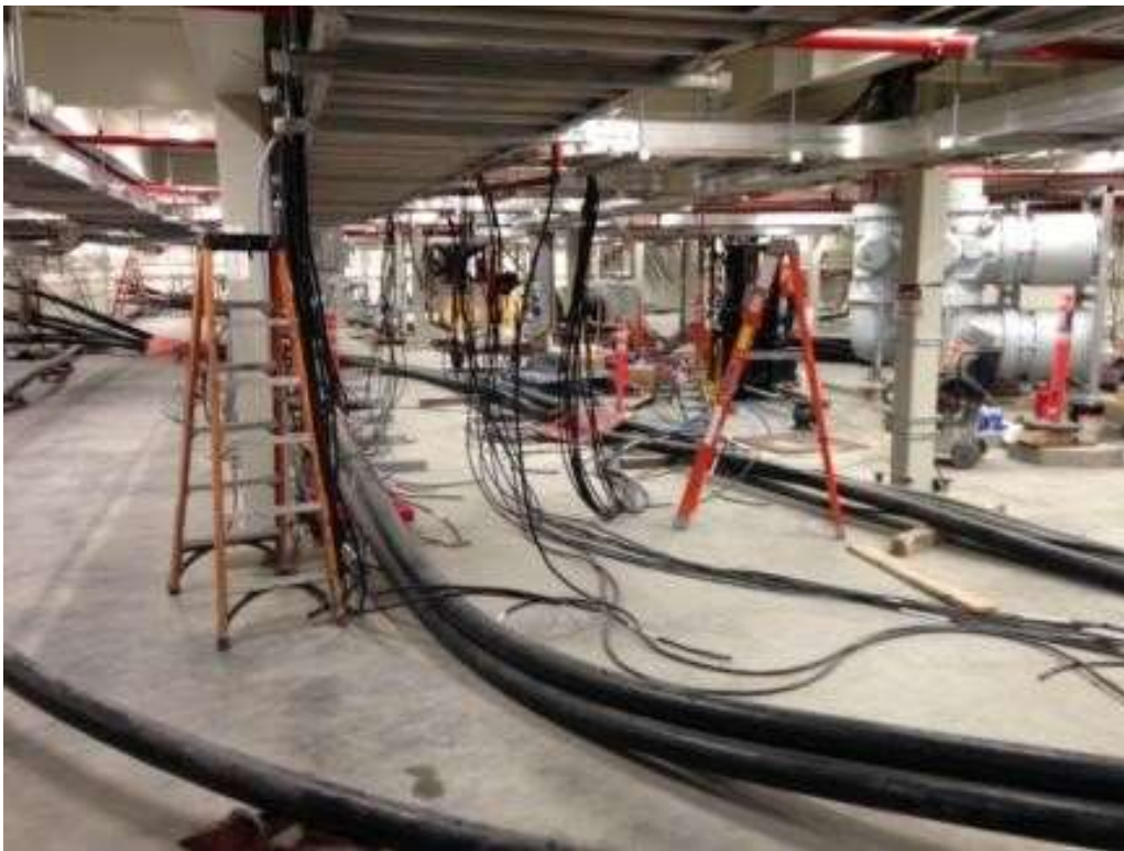
Figure 4: CCE electrical work in GIS building basement in Potrero Switchyard, July 6, 2016. Photo courtesy of PG&E.
