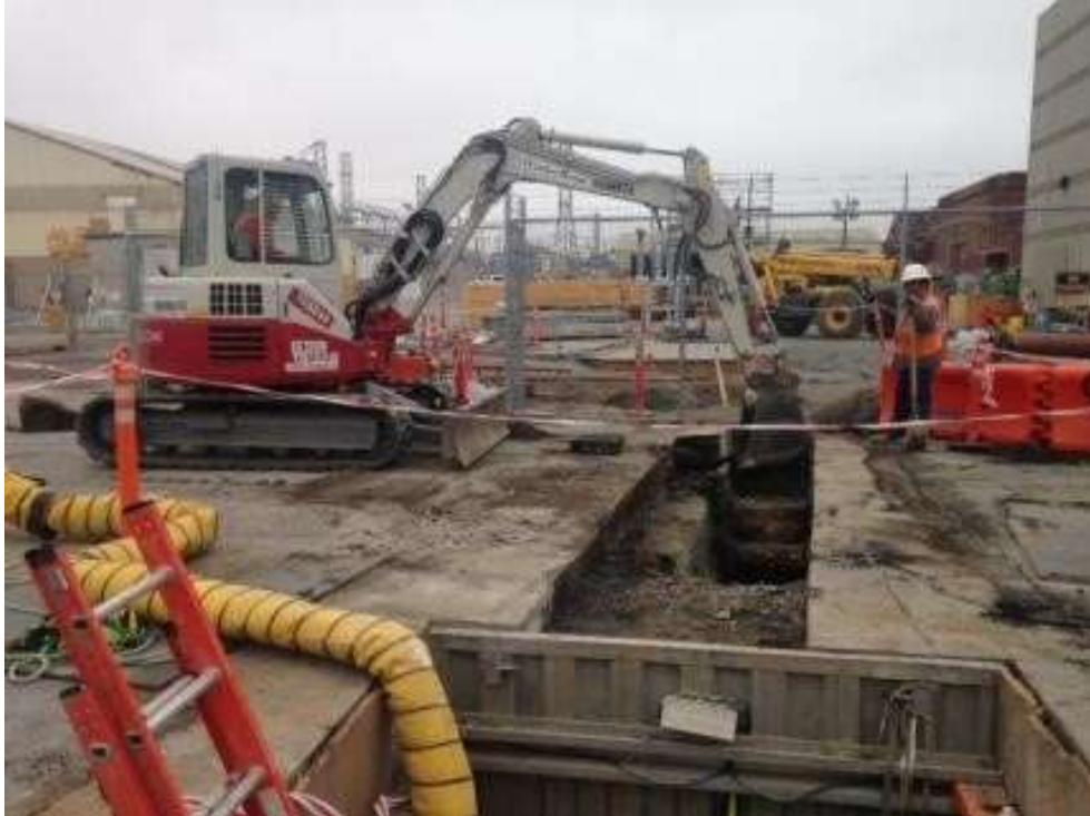
Figure 2: APEC excavated for the water and sewer line tie-in on 23 rd Street, July 6, 2016. Photo courtesy of PG&E.
