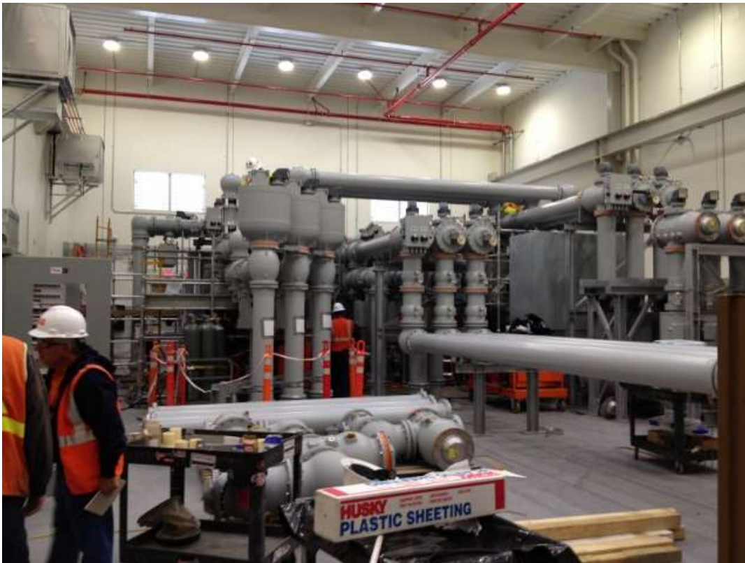
Figure 4: CCE installing infrastructure and electrical work in GIS building in Potrero Switchyard, July 12, 2016.
