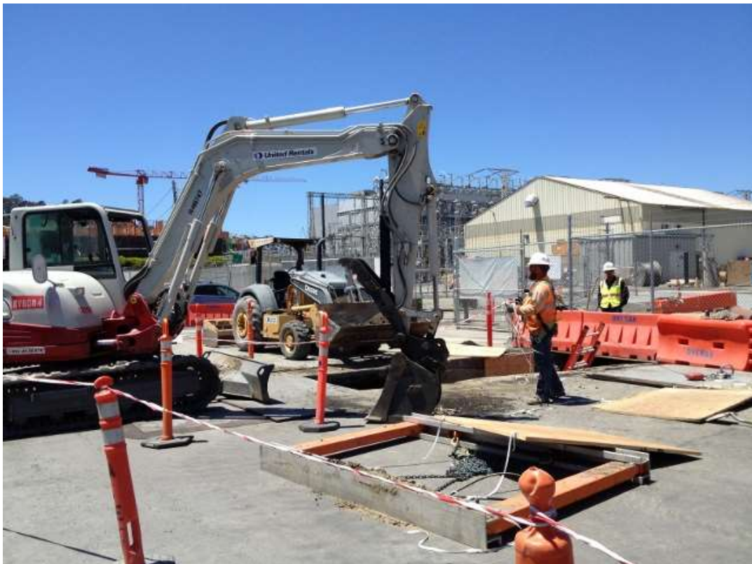
Figure 2: APEC conducting water and sewer line tie-in work on 23 rd Street, July 12, 2016.
