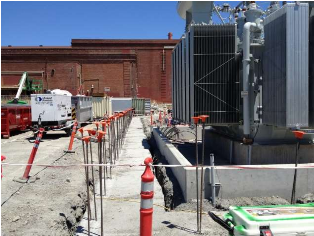
Figure 3: Overaa installing rebar and forms for perimeter wall at Potrero Switchyard, July 12, 2016.
