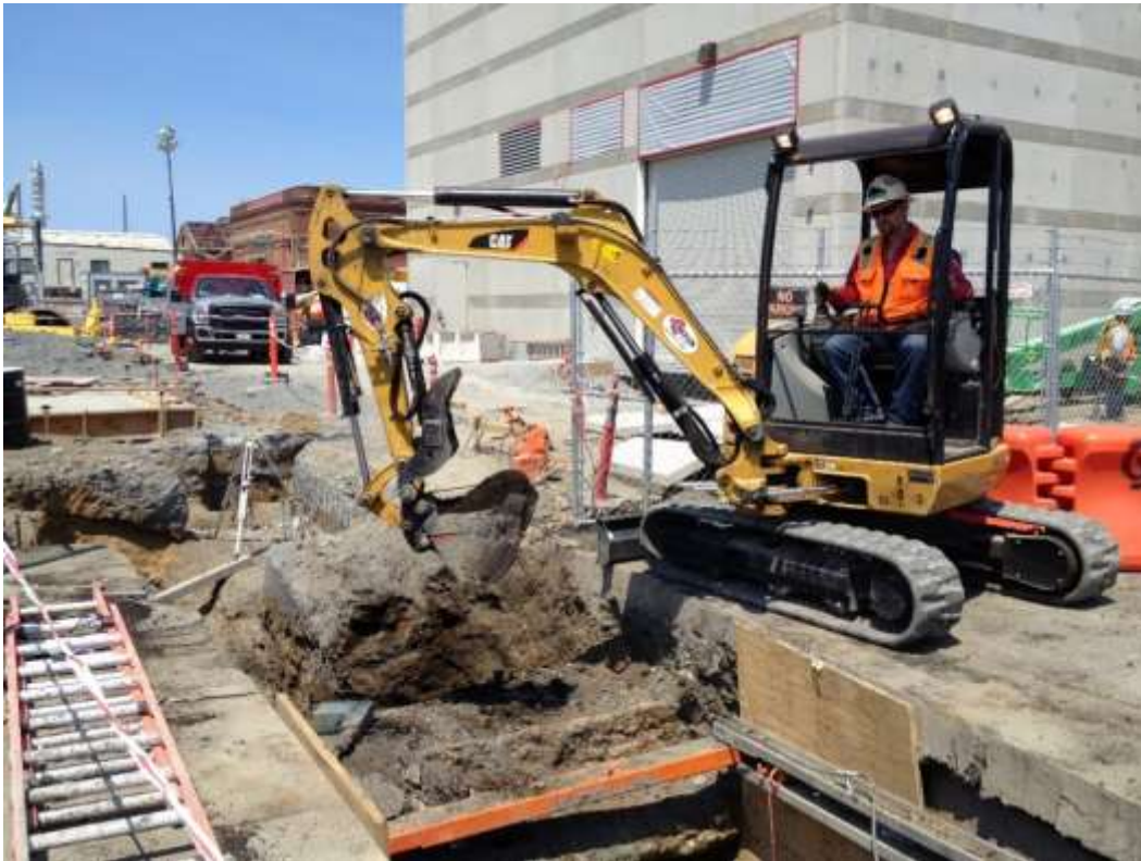
Figure 2: APEC conducting water and sewer line tie-in work on 23 rd Street, July 26, 2016.
