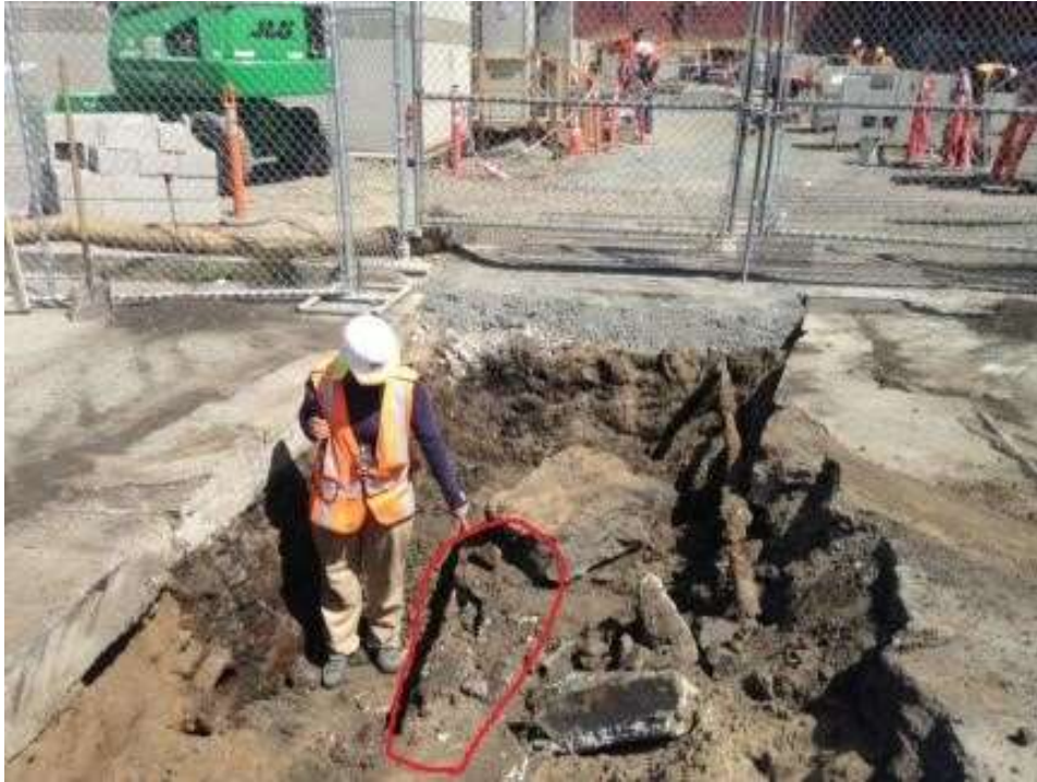
Figure 1: APEC excavated for the water and sewer line tie-in in front of the easternmost gate south of the Switchyard on 23 rd Street where an old redwood pipe was uncovered, August 2, 2016. Photo courtesy of PG&E.
