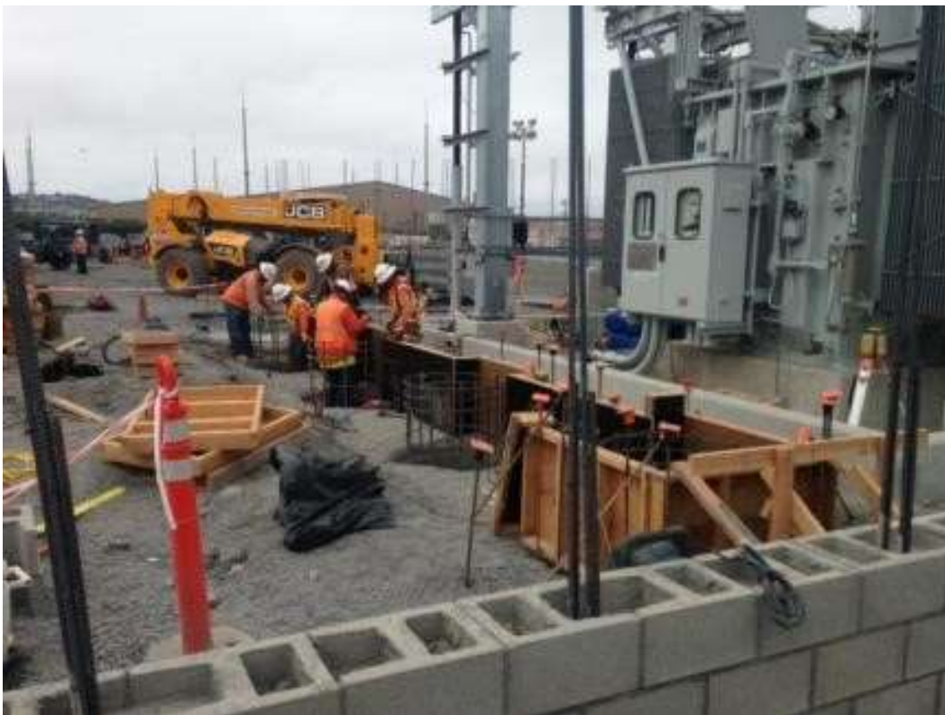
Figure 4: Spencer Masonry installed rebar, bricks, and mortar for the perimeter wall, August 2, 2016. Photo courtesy of PG&E.
