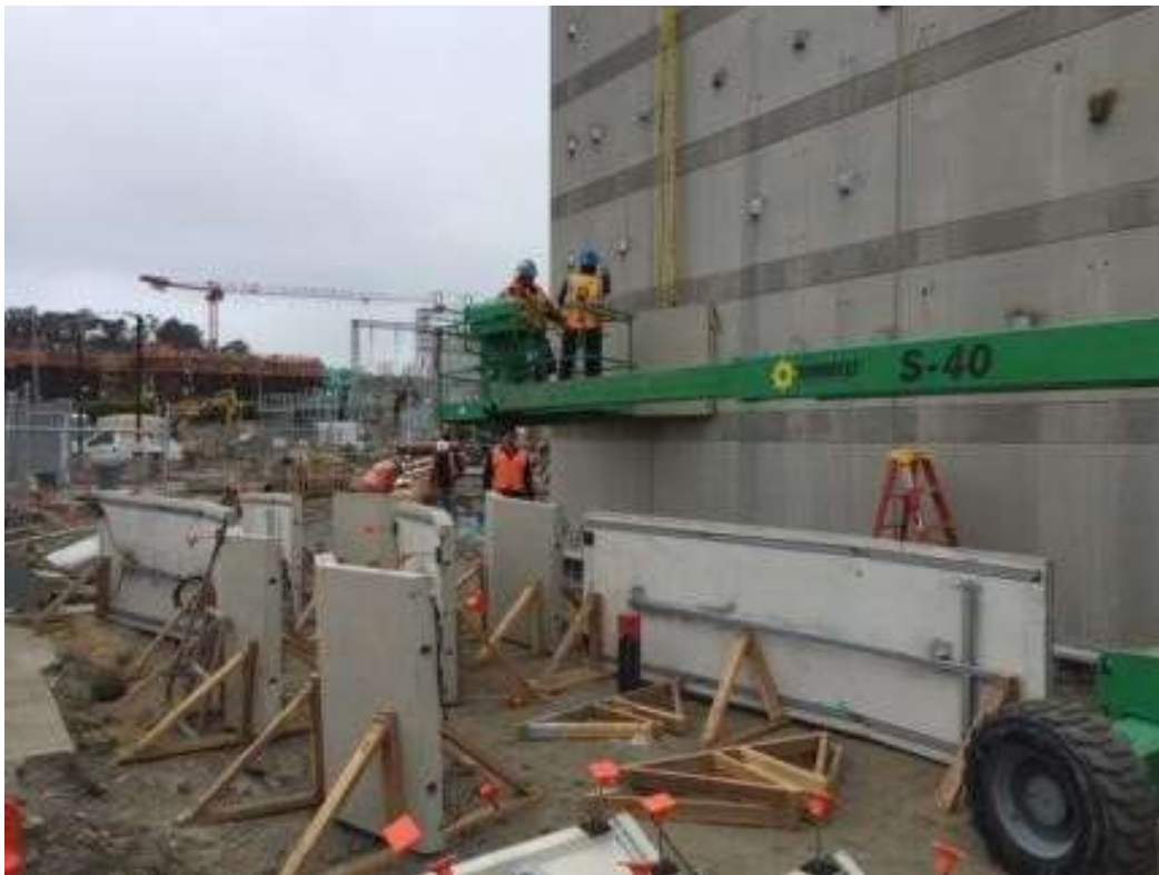
Figure 3: Overaa drilled the outside walls of the GIS building, installed metal hangers, and welded hangers for the installation of the architectural panels, August 4, 2016. Photo courtesy of PG&E.
