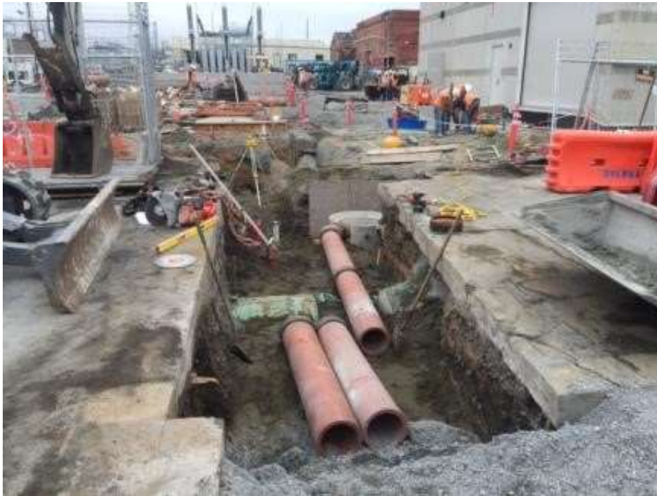
Figure 2: APEC installed a storm drain in the excavation for the water and sewer tie-in in front of the westernmost yard gate south of the switchyard on 23 rd Street, August 4, 2016. Photo courtesy of PG&E.
