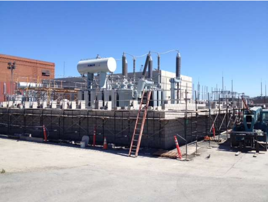
Figure 4: Spencer Masonry installed rebar, bricks, and mortar for the perimeter wall, August 9, 2016.
