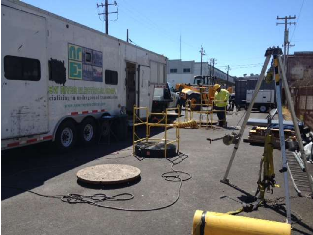
Figure 1: Sumitomo and NRE installed racking, cut cable, and prepared to splice cable in the transition vault on 23 rd Street, August 9, 2016.
