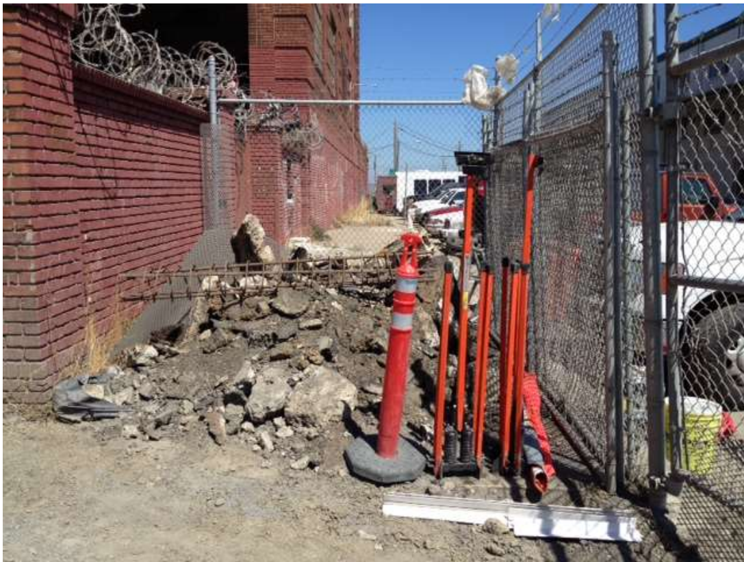
Figure 5: Stockpile of rubble and soil at the southeast corner of the Switchyard to be removed or covered, August 9, 2016.
