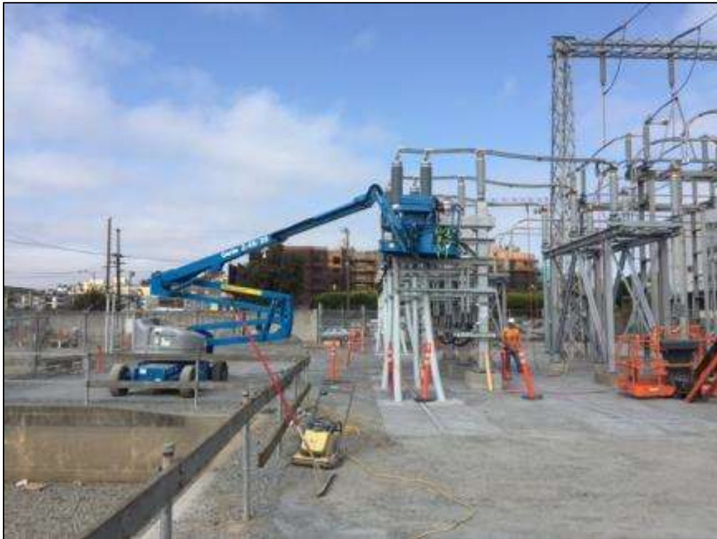
CCE conducting electrical work on 115 kV bus in Potrero Substation, August 18, 2016. Photo courtesy of PG&E.
