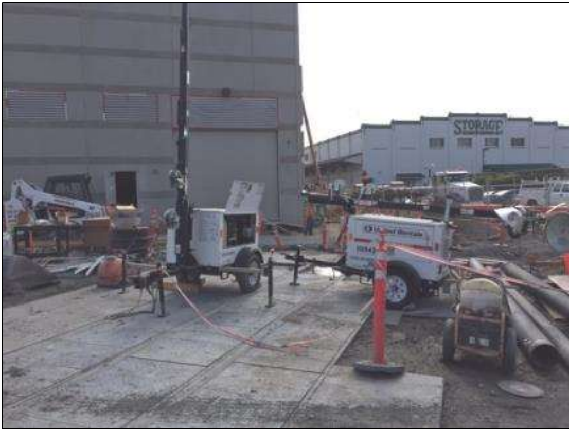
Lighting structures without containment in Potrero Switchyard, August 18, 2016. Photo courtesy of PG&E.
