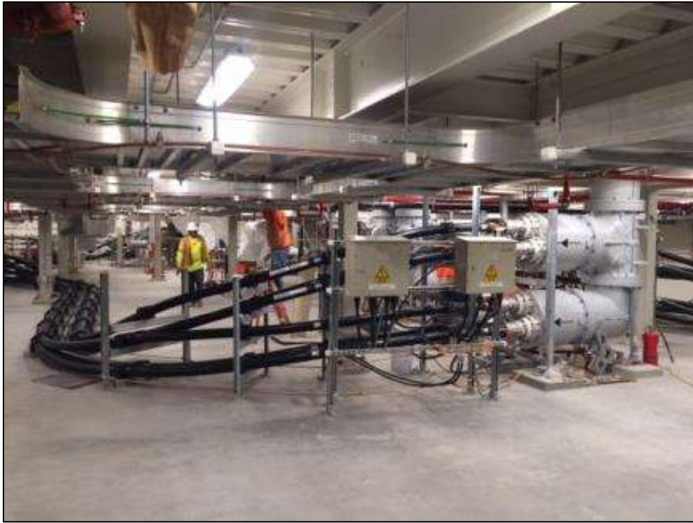
Nexans working on wire in GIS basement at Potrero Switchyard, August 15, 2016. Photo courtesy of PG&E.
