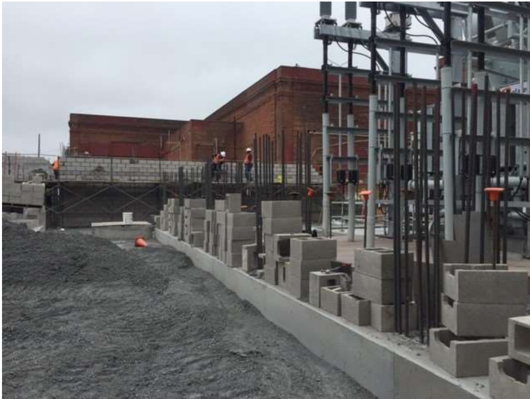
Figure 3 - Spencer Masonry building perimeter wall in Potrero Switchyard, August 22, 2016. Photo courtesy of PG&E.
