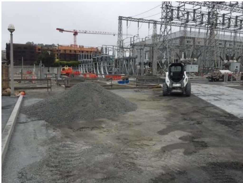
Figure 4 - APEC backfilling and compacting base rock in Potrero Substation, August 22, 2016. Photo courtesy of PG&E.
