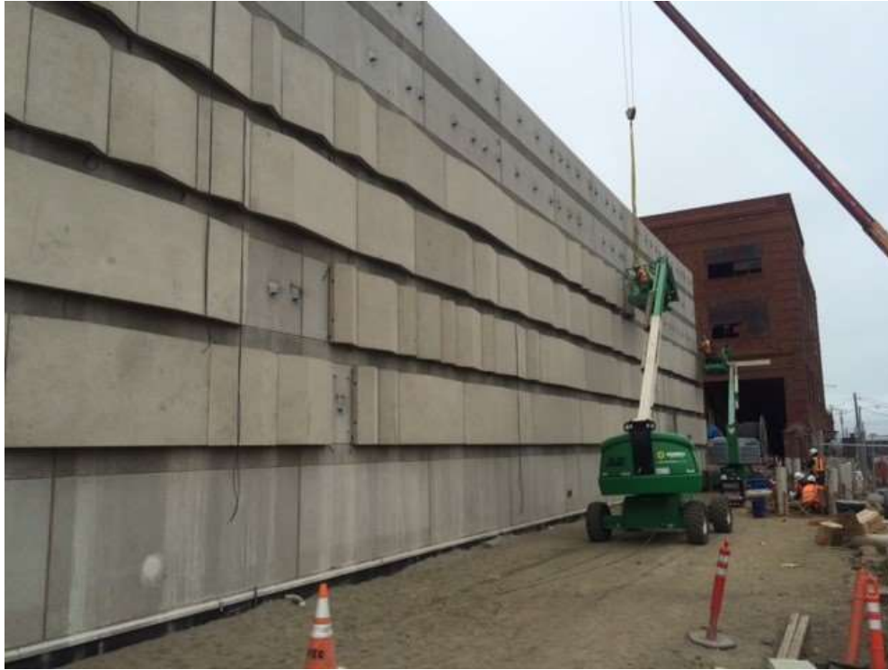
Figure 1 - Overaa installing architectural tiles on GIS building at Potrero Switchyard, August 25, 2016. Photo courtesy of PG&E.
