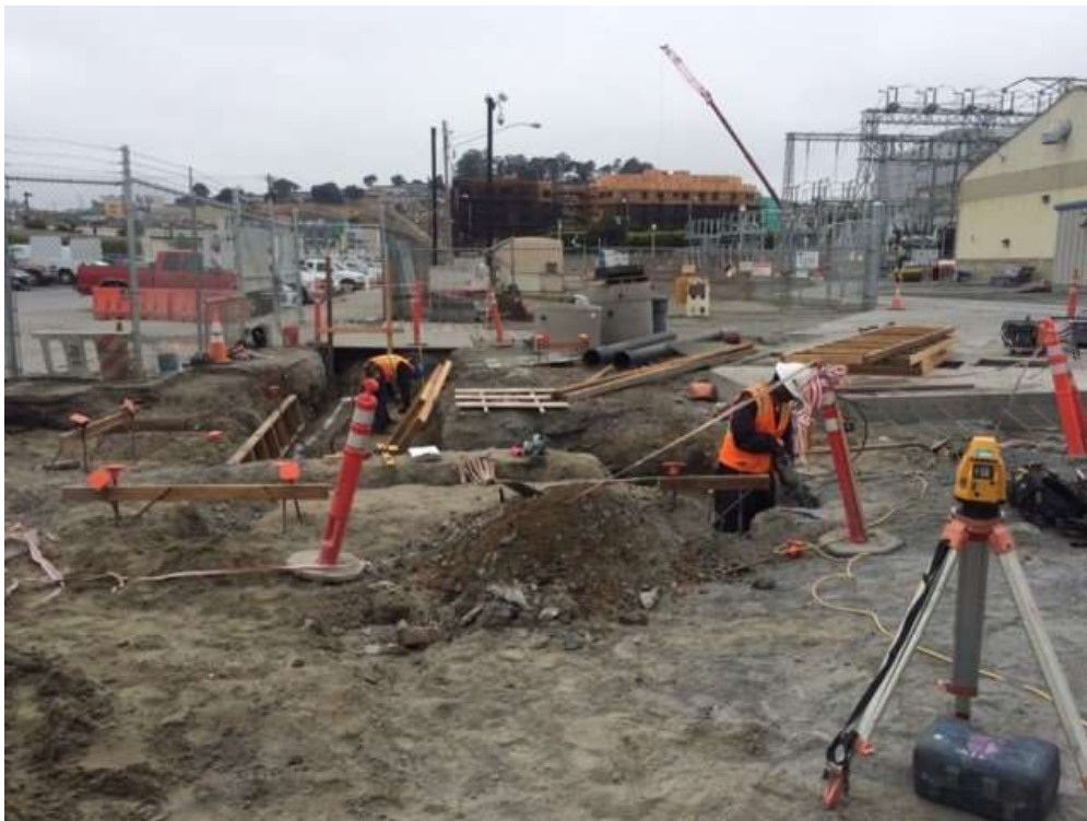
Figure 2 - Overaa installed wall footings in Potrero Switchyard, August 25, 2016. Photo courtesy of PG&E.
