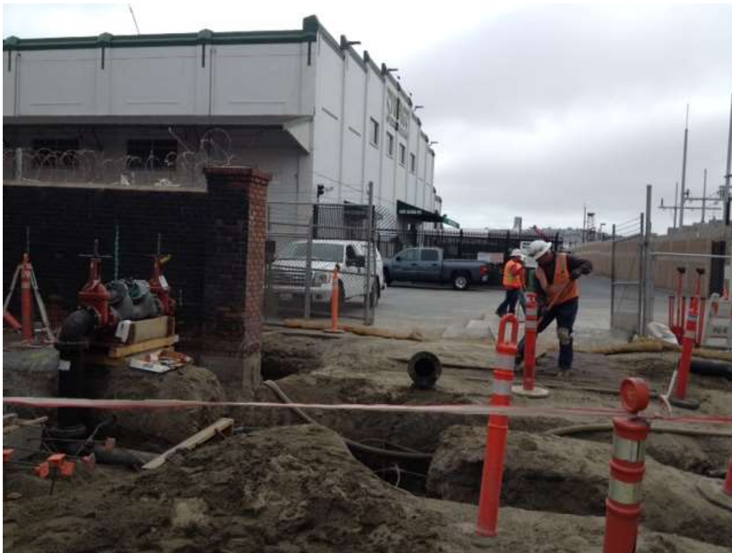
Figure 4 - APEC excavated and installed water/sewer pipe near SE corner of the GIS building, September 1, 2016.
