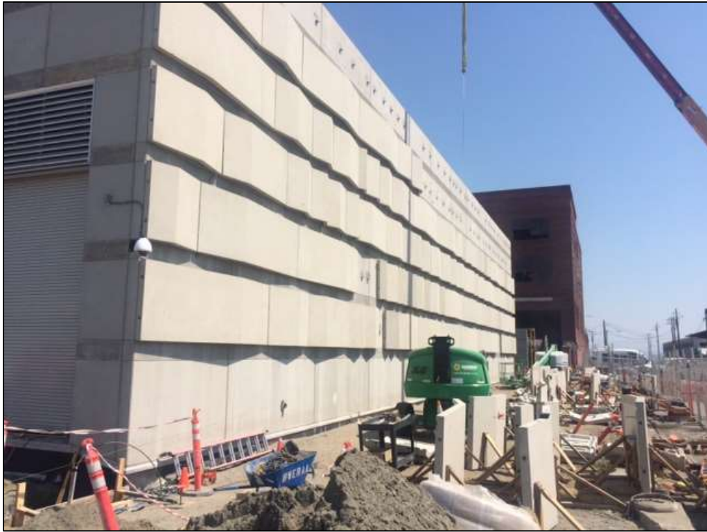
Figure 1 - Overaa installing architectural tiles on GIS building at Potrero Switchyard, September 6, 2016. Photo courtesy of PG&E.
