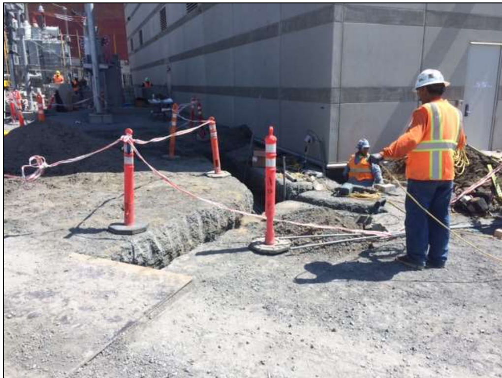
Figure 2 – Overaa installed gate footings outside of the GIS building, September 8, 2016. Photo courtesy of PG&E
