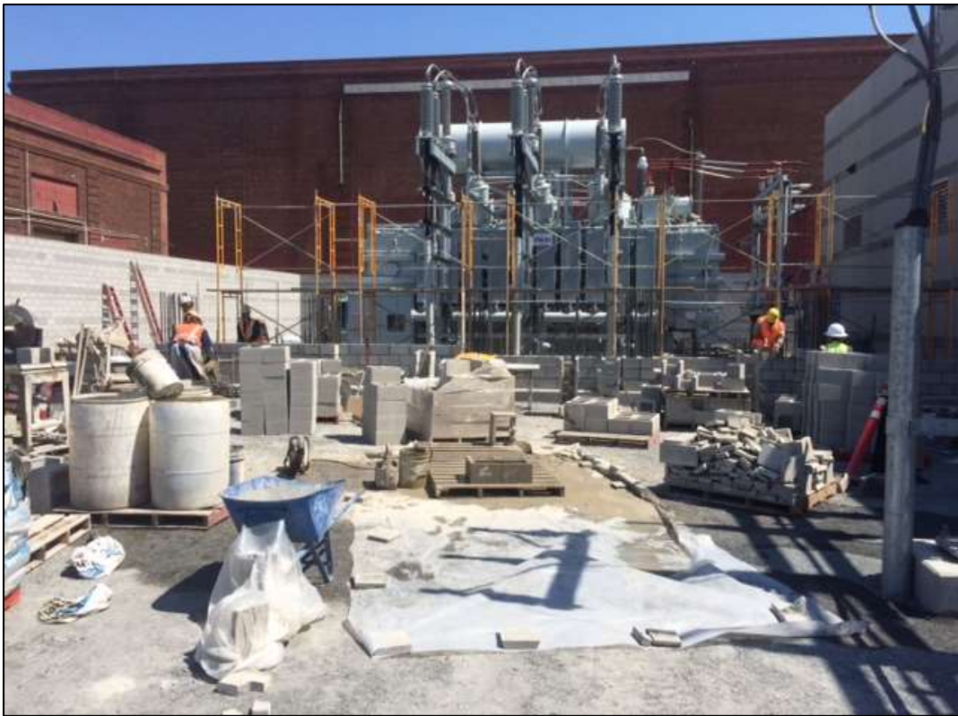
Figure 3 - Spencer Masonry building fire wall around transformer, September 8, 2016. Photo courtesy of PG&E
