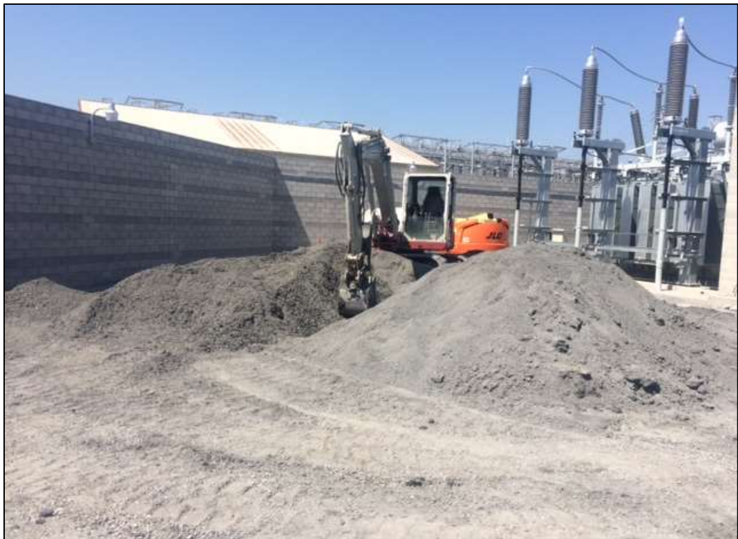
Figure 4 - APEC backfilled and compacted around the GIS building, September 6, 2016. Photo courtesy of PG&E.
