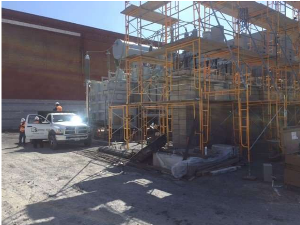
Figure 2 – Spencer Masonry building fire wall around transformer, September 15, 2016. Photo courtesy of PG&E.
