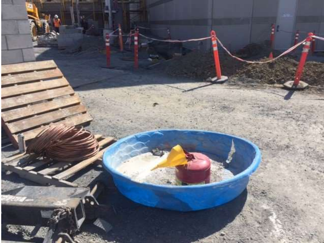
Figure 4 – Unlined kiddie pool for concrete washout with cracks, September 15, 2016. Photo courtesy of PG&E.
