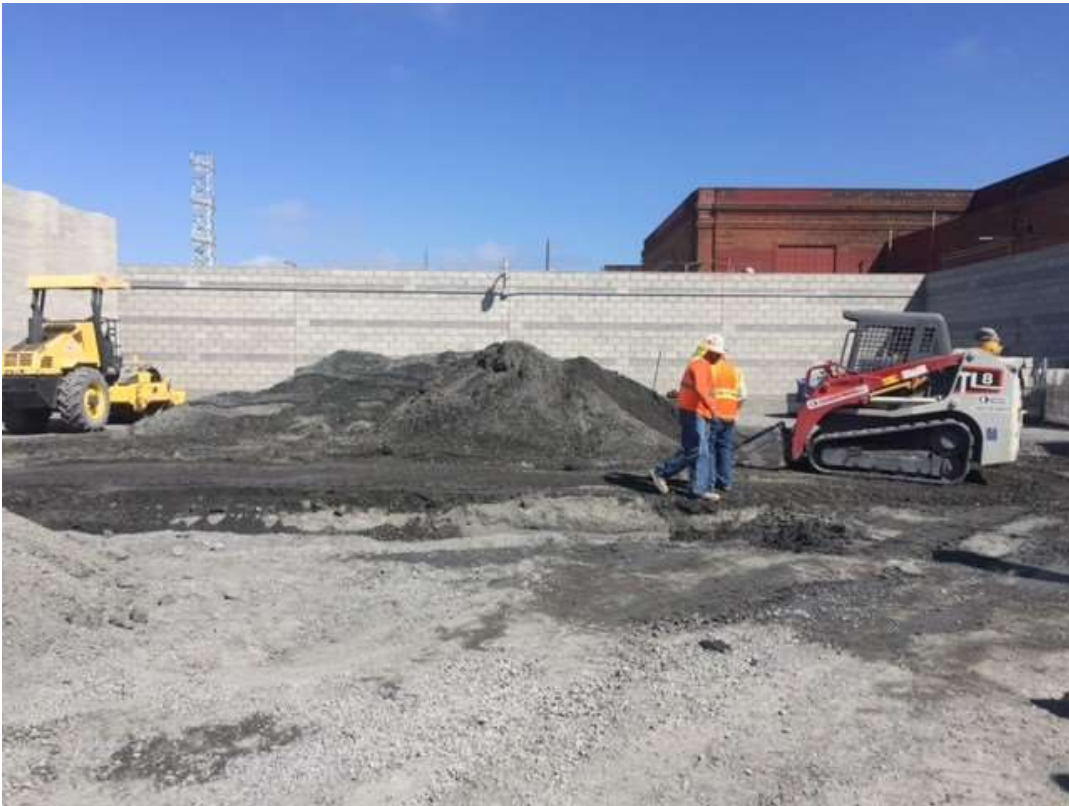
Figure 3 - APEC backfilled and compacted around the GIS building, September 15, 2016. Photo courtesy of PG&E.
