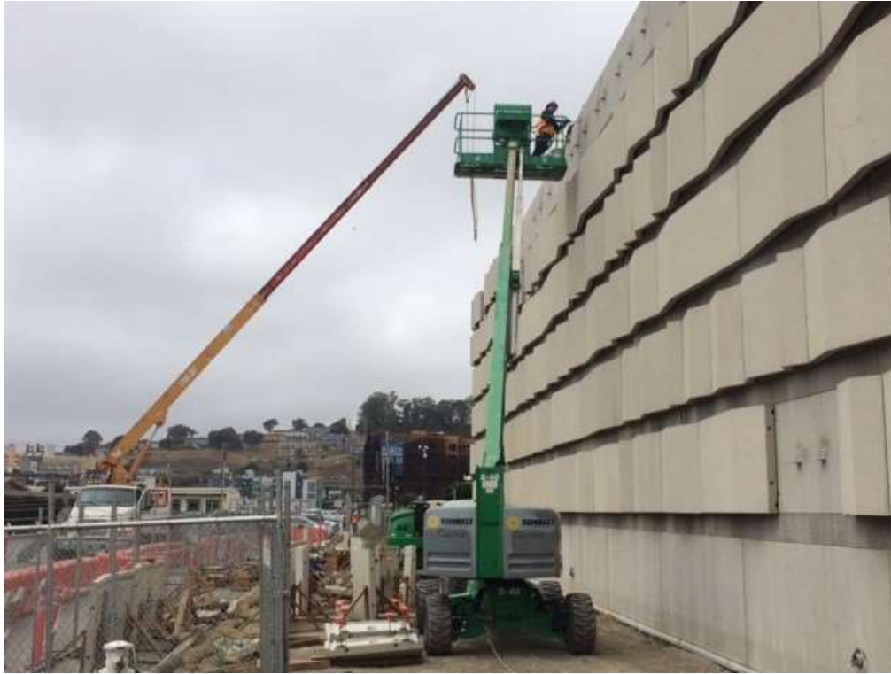
Figure 1 - Overaa installing architectural tiles on GIS building at Potrero Switchyard, September 12, 2016. Photo courtesy of PG&E.
