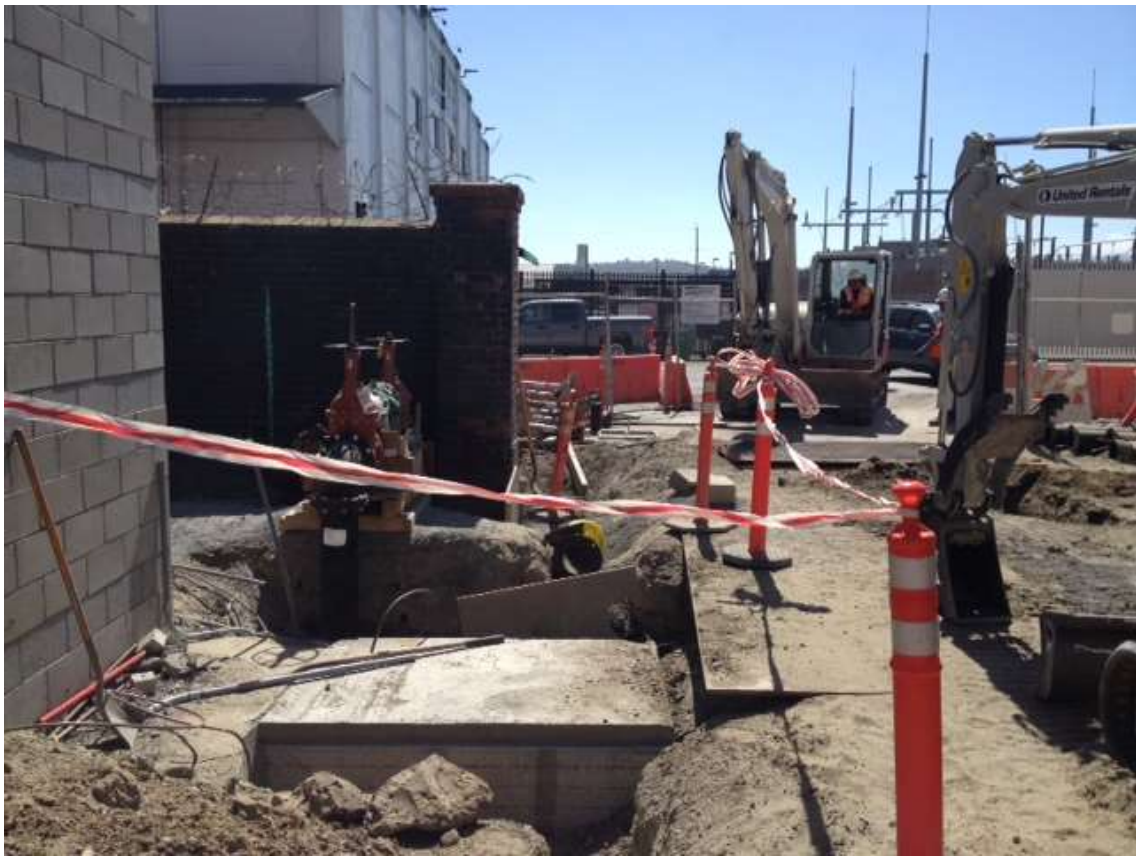
Figure 3 - APEC excavated and installed conduit near southeast corner of GIS building for water and sewer tie-in, September 21, 2016.
