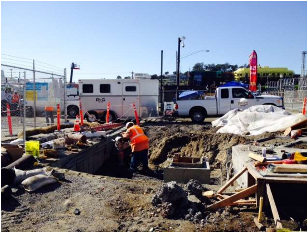
Figure 2 - APEC backfilling around the water and sewer tie-in near the southwest corner of the GIS building, October 26, 2016.
