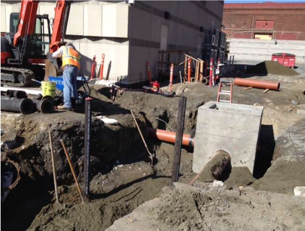
Figure 1 – APEC backfilling around the water and sewer tie-in near the southeast corner of the GIS building, October 26, 2016.
