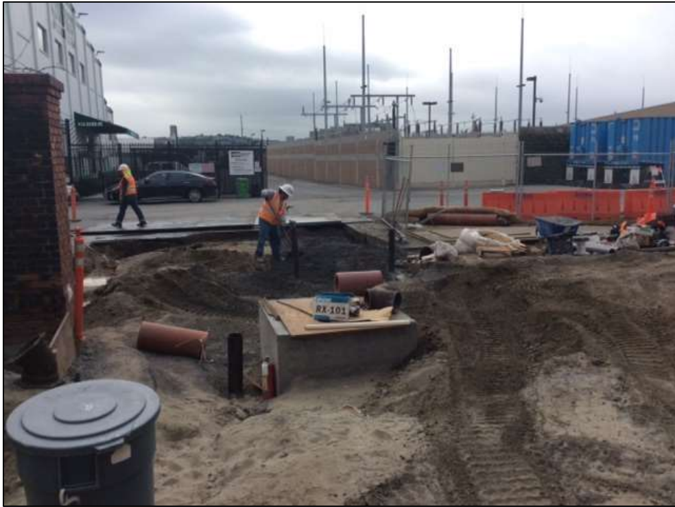
Figure 1 – APEC backfilling in southwest corner of Switchyard, November 15, 2016. Photo courtesy of PG&E.
