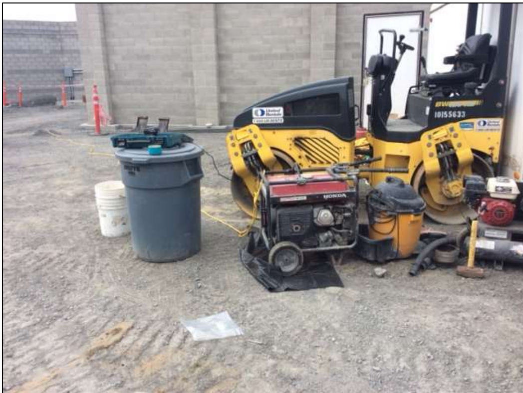
Figure 4 – Generator with insufficient containment in the Switchyard, November 15, 2016. Photo courtesy of PG&E.
