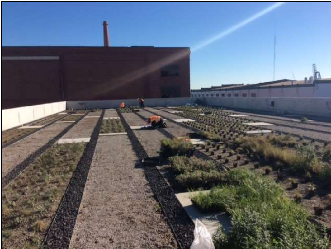
Figure 3 – Planting vegetation on the roof of the GIS building, November 18, 2016. Photo courtesy of PG&E.
