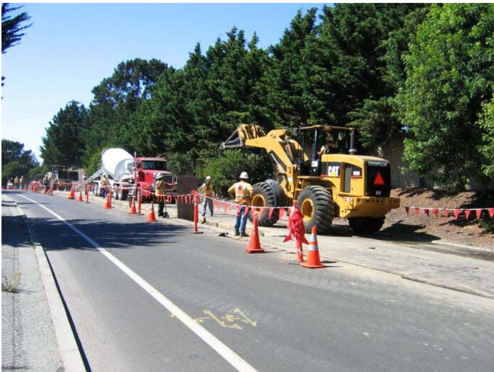
Figure 2 – Crews conducting trenching activities on Skyline Boulevard south of Manhole #33, Segment 2 Underground, August 23, 2005
