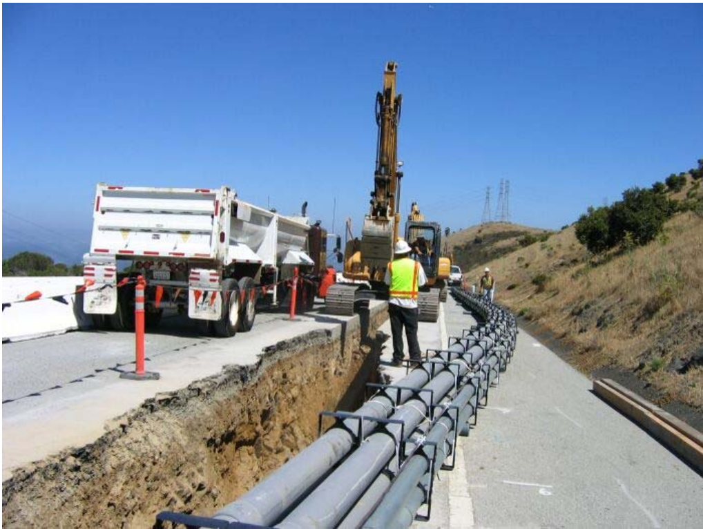
Figure 5 – Trenching activities and conduit installation on east side of San Bruno Mountain along Guadalupe Canyon Parkway, Segment 5, August 11, 2005.
