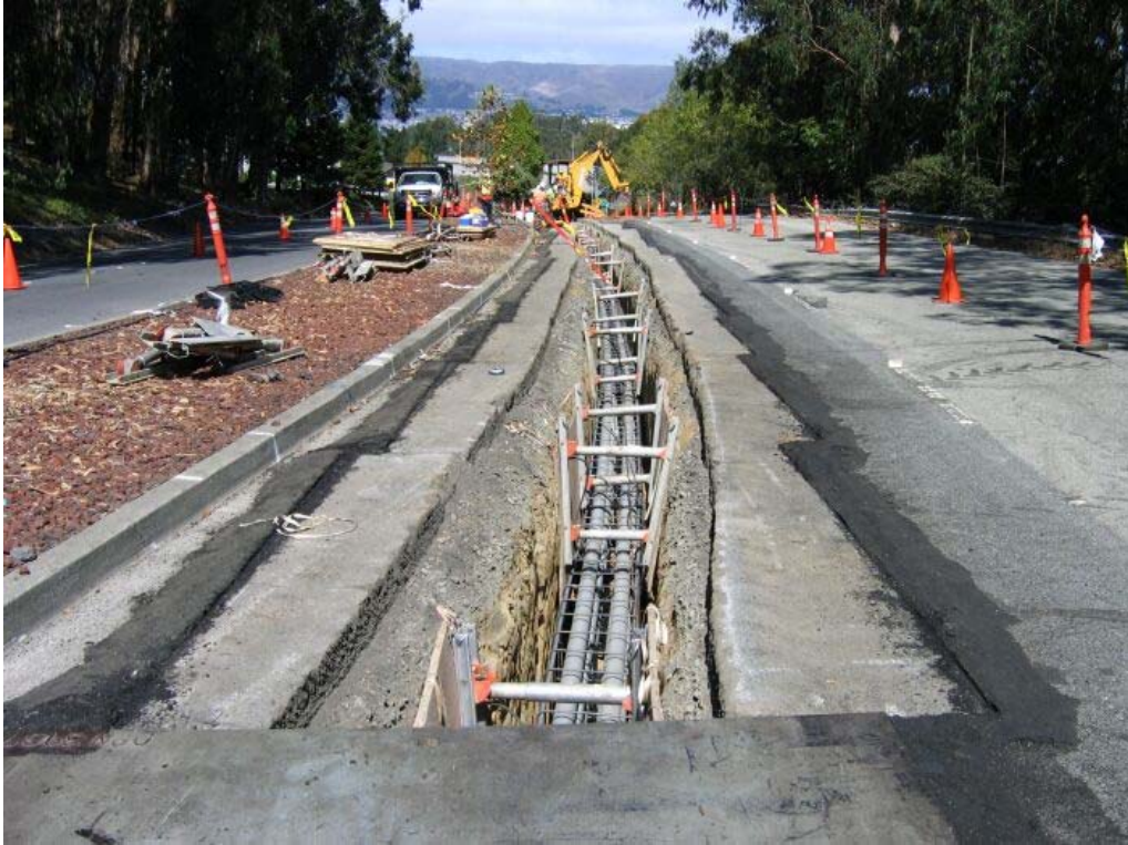
Figure 3 – Conduit installation between Manhole #41 and Manhole #42 on San Bruno Avenue, Segment 3, September 13, 2005
