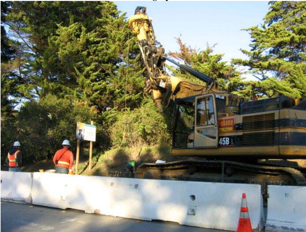
Figure 1 – Crews finishing the foundation for the transition tower on the north side of Crystal Springs Dam, Segment 1, December 6, 2005.
