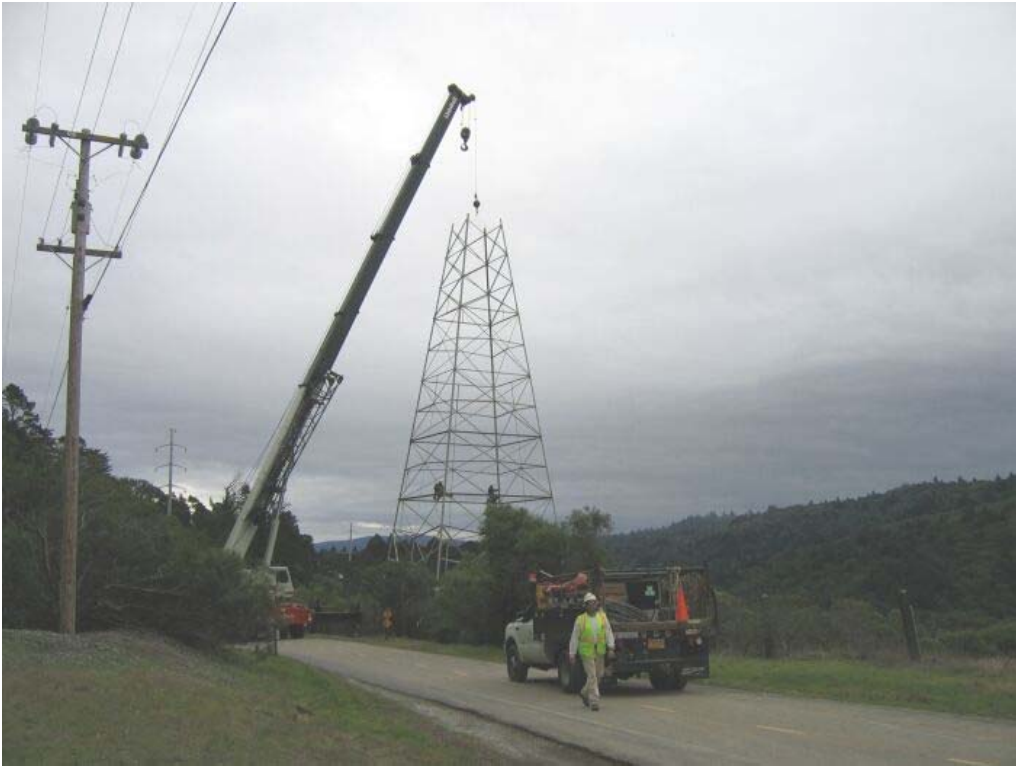
Figure 4 – Crews removing the old lattice #74 tower with a crane, Segment 2 Overhead, December 20, 2005.
