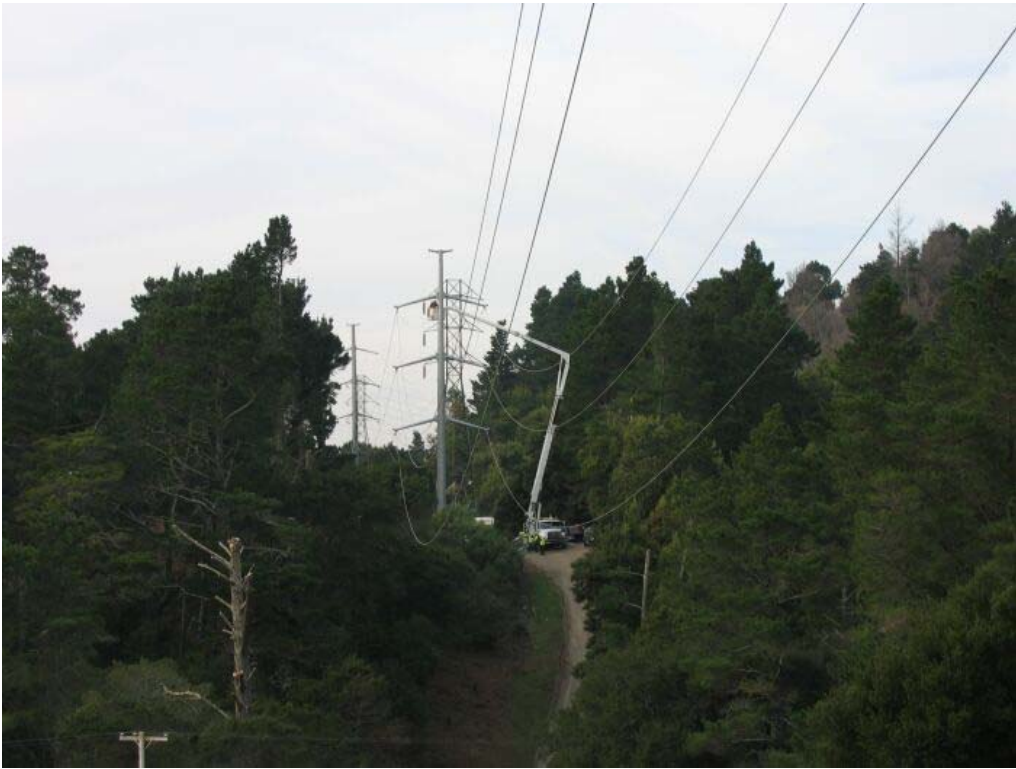
Figure 3 – Crews removing wire from old tower and transferring it to new Tower #71, Segment 2 Overhead, December 14, 2005.
