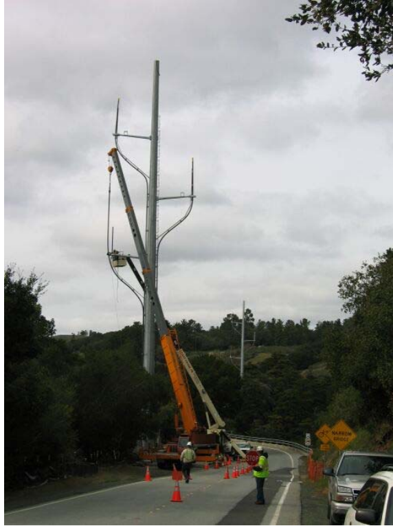
Figure 1 – Cable being pulled up tower on the south side of Crystal Springs Dam, Segment 1, March 22, 2006.
