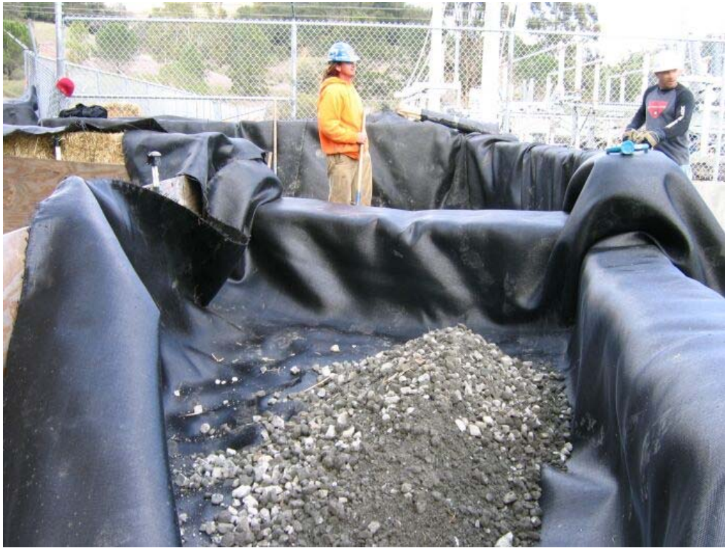
Figure 3 – Crews building a temporary retention basin in the right-of-way at the northwest corner of the substation to catch storm water run-off, Jefferson Substation, March 9, 2006.
