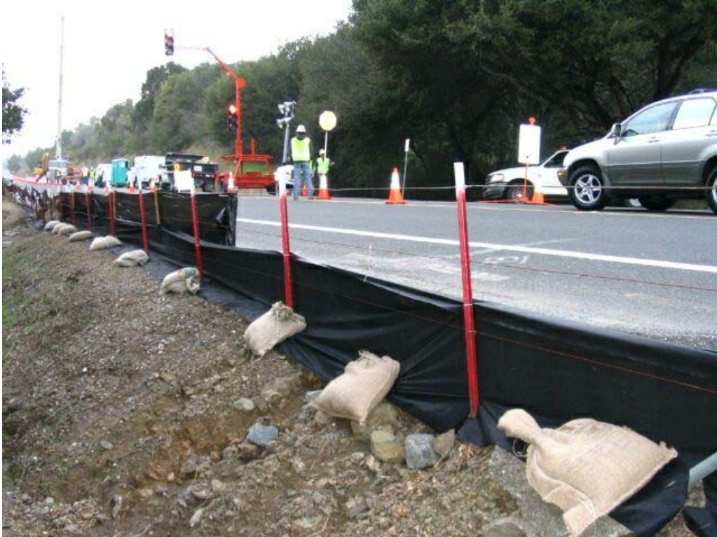
Figure 1 – Exclusion fencing along west side of Cañada Road just south of Manhole #9 on Segment 1, January 24, 2005.
