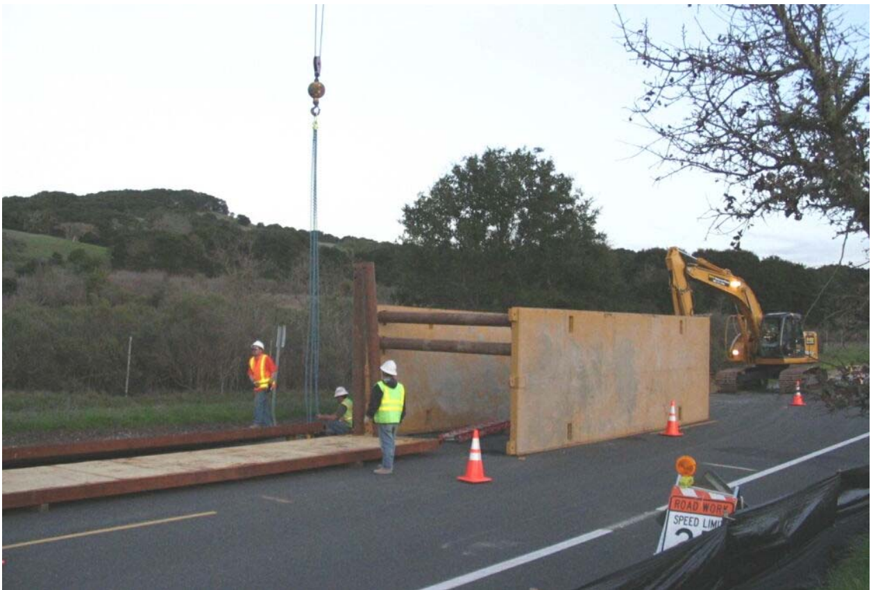
Figure 2 – Crews setting up shoring at MH #7 along Cañada Road on Segment 1, January 31, 2005.
