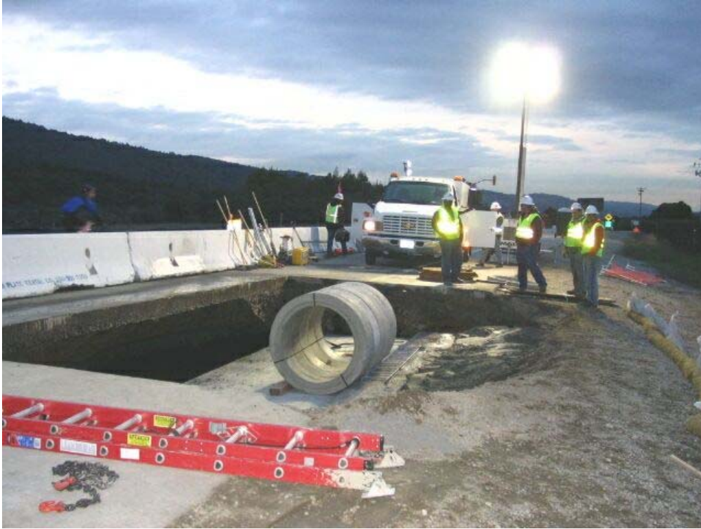
Figure 1 – Manhole #3 on Cañada Road, Segment 1, February 8, 2005. Vault installed and ready to excavate cave-in on west side of vault.
