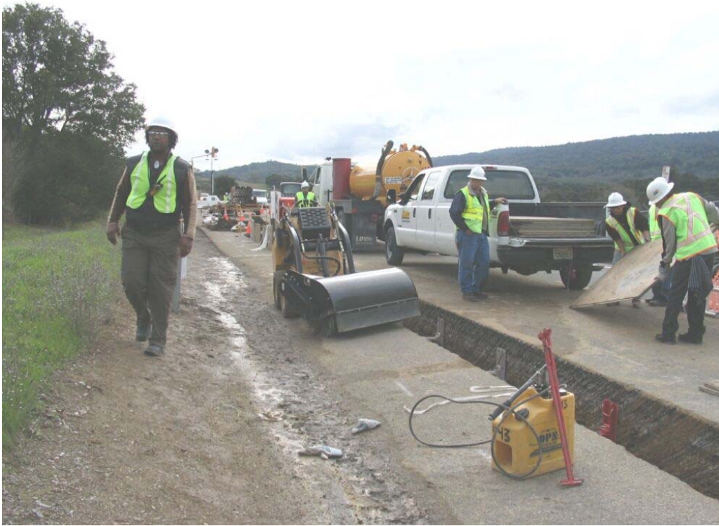
Figure 3 – Spoil spill due to trenching activities at Station #106+00 on Cañada Road, Segment 1, February 8, 2005.
