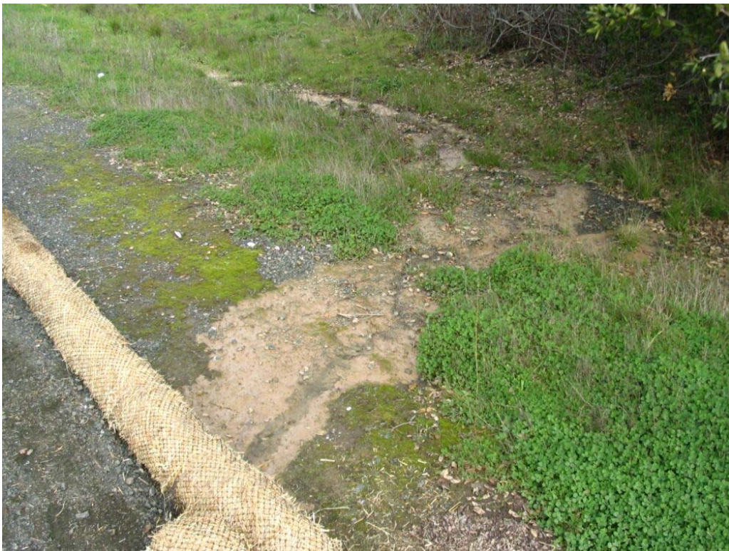
Figure 4 – Spoil spill into vegetated drainage at Station #108+00 on Cañada Road, Segment 1, February 8, 2005
