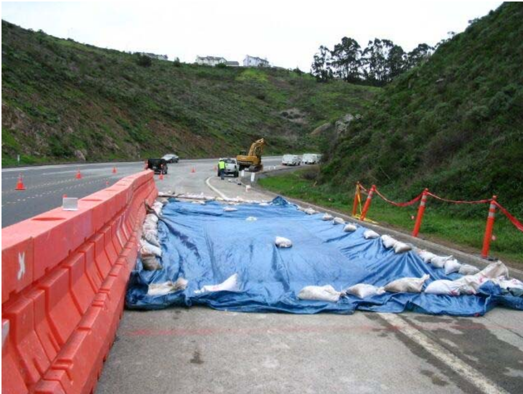
Figure 5 – Manhole #67 covered and sandbagged to prevent stormwater from entering area, Segment 5, February 17, 2005
