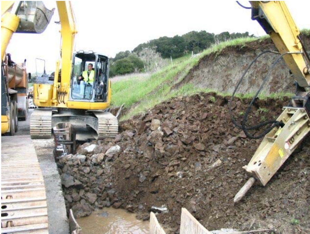
Figure 3 – Hillside failure along trenching at approximately Station #84+00 on Cañada Road, Segment 1, March 3, 2005
