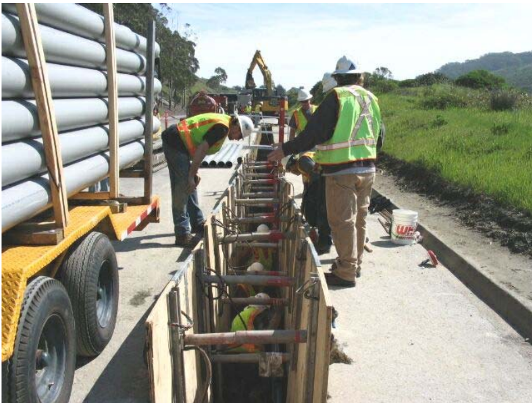
Figure 4 – Crews installing conduit east of Manhole #68 on Guadalupe Canyon Parkway, Segment 5, March 7, 2005
