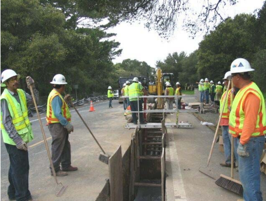
Figure 1 – Crews installing conduit on Cañada Road North of Edgewood intersection, Segment 1, March 16, 2005.
