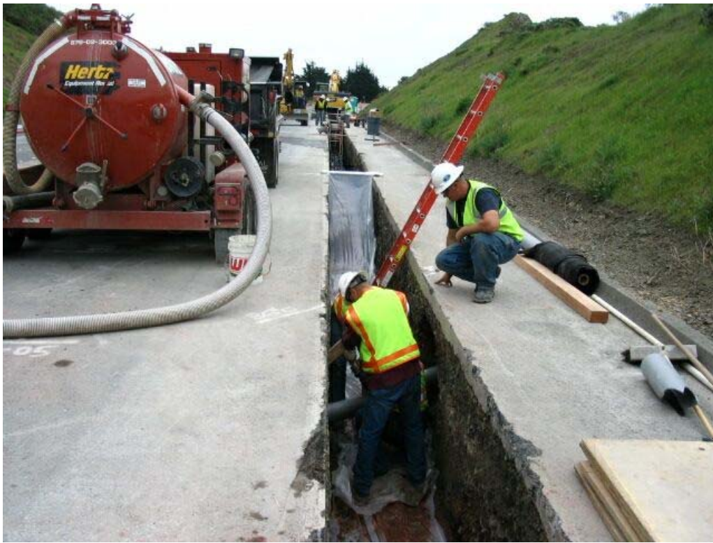
Figure 5 – Crews fixing culvert in trench east of Manhole #68 on Guadalupe Canyon Parkway, Segment 5, March 17, 2005.
