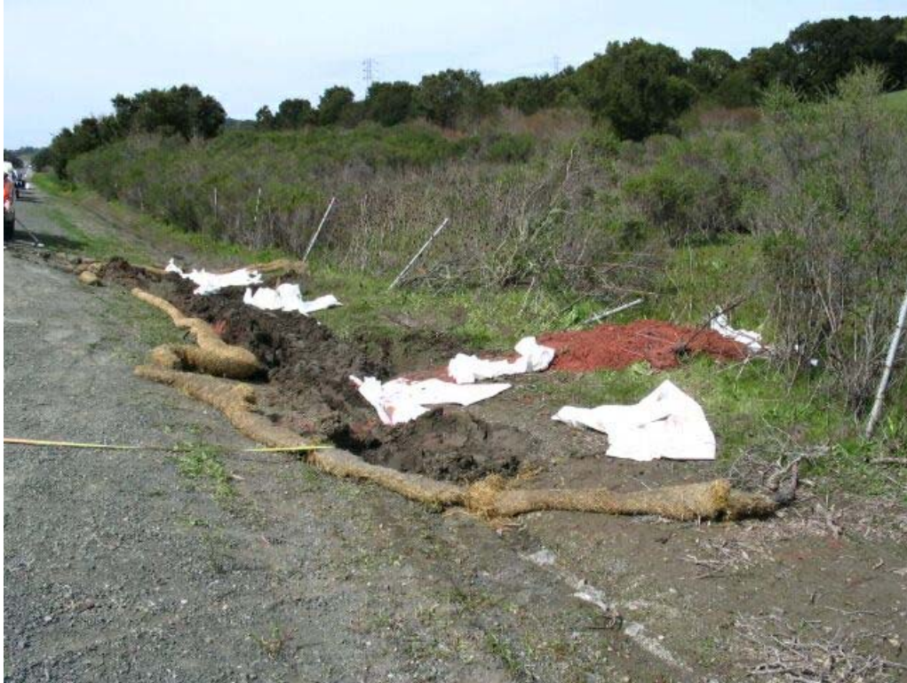
Figure 3 – Area where concrete truck flipped over and spilled concrete (red material) and hydraulic fluid along side of Cañada Road, Segment 1, March 16, 2005.
