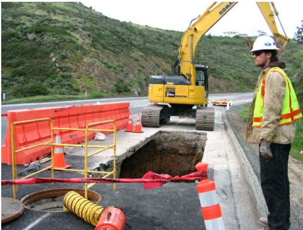
Figure 4 – Crews working at stub-outs on east side of Manhole #67 on Guadalupe Canyon Parkway, Segment 5, March 16, 2005.
