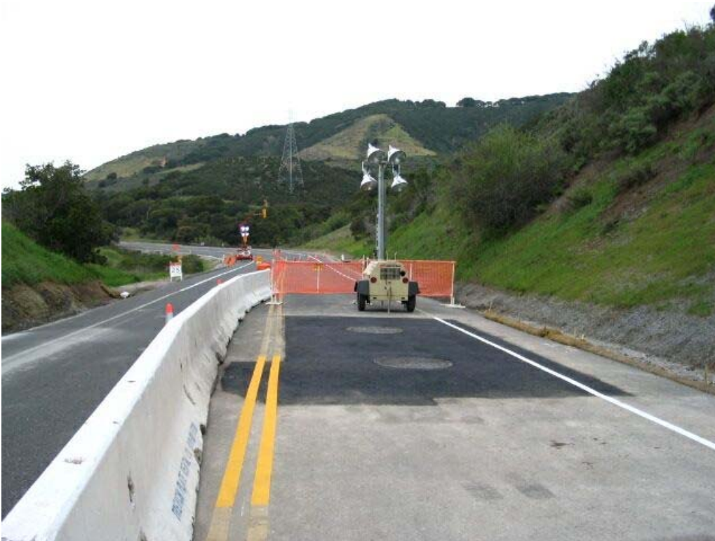
Figure 2 – Manhole #12 paved over, Cañada Road, Segment 1, March 16, 2005.
