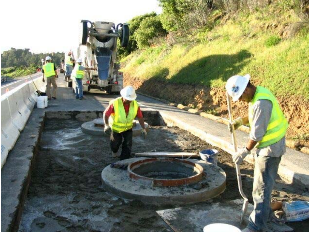
Figure 3 – Crews getting ready to pour more cement slurry at Manhole #11 on Cañada Road, Segment 1, March 30, 2005.
