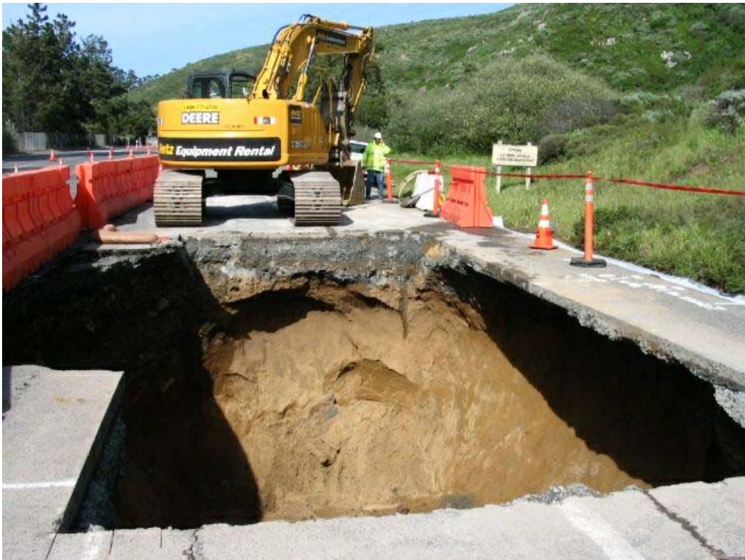
Figure 4 – Manhole #66 vault pit having cave-in issues on Guadalupe Canyon Parkway, Segment 5, March 28, 2005.
