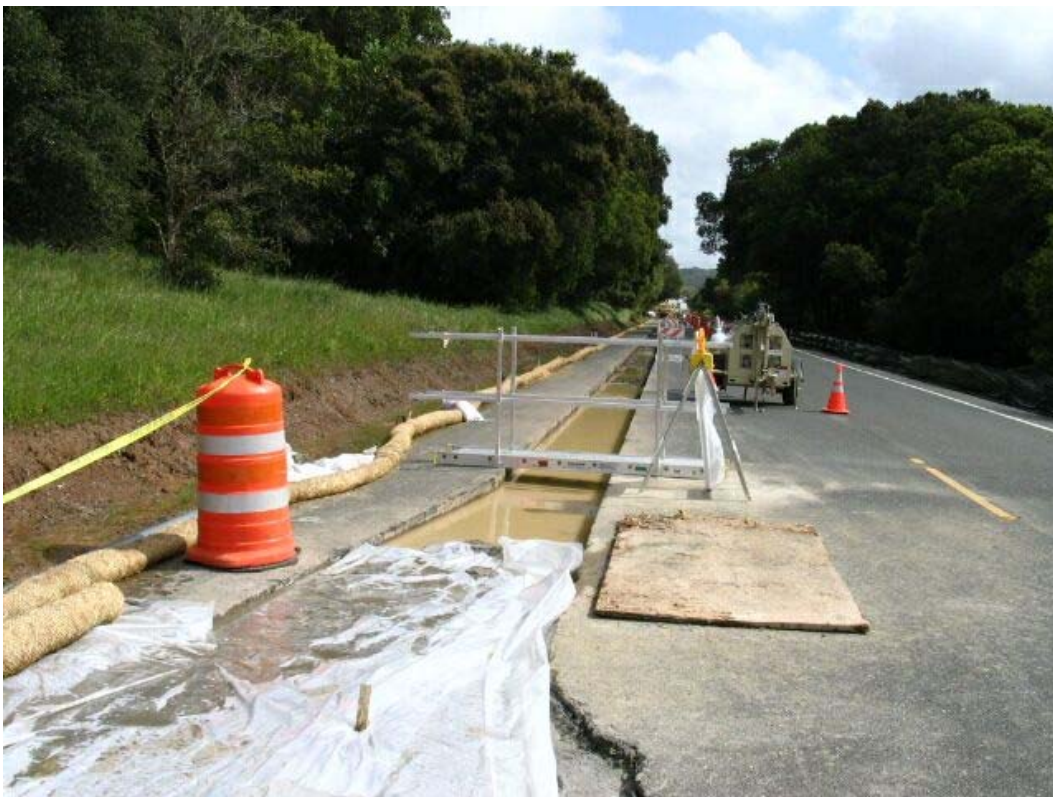
Figure 2 – Water in trench south of Manhole #5 on Cañada Road, Segment 1, March 29, 2005.
