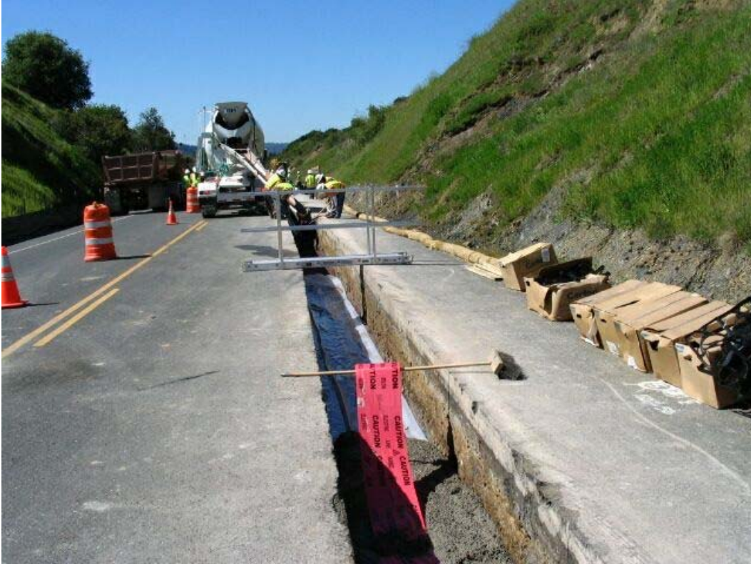
Figure 1 – Crews conducting trenching activities between Manholes #10 and #11 on Cañada Road, Segment 1, April 5, 2005.
