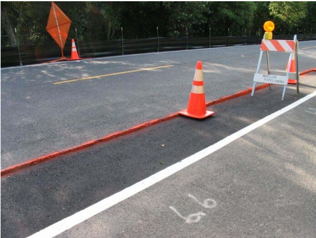
Figure 2 – Area where trench sank between Manholes #4 and #5 on Cañada Road, Segment 1, April 12, 2005.
