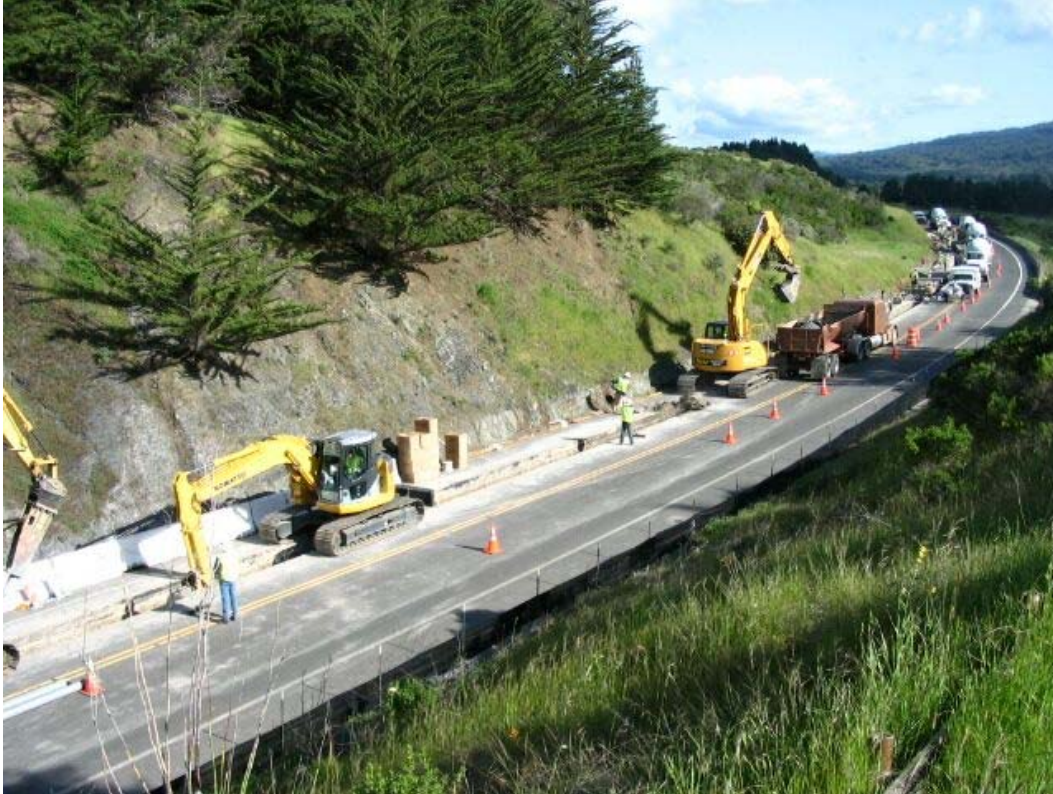
Figure 1 – Crews conducting trenching activities between Manholes #11 and #12 on Cañada Road, Segment 1, April 13, 2005.
