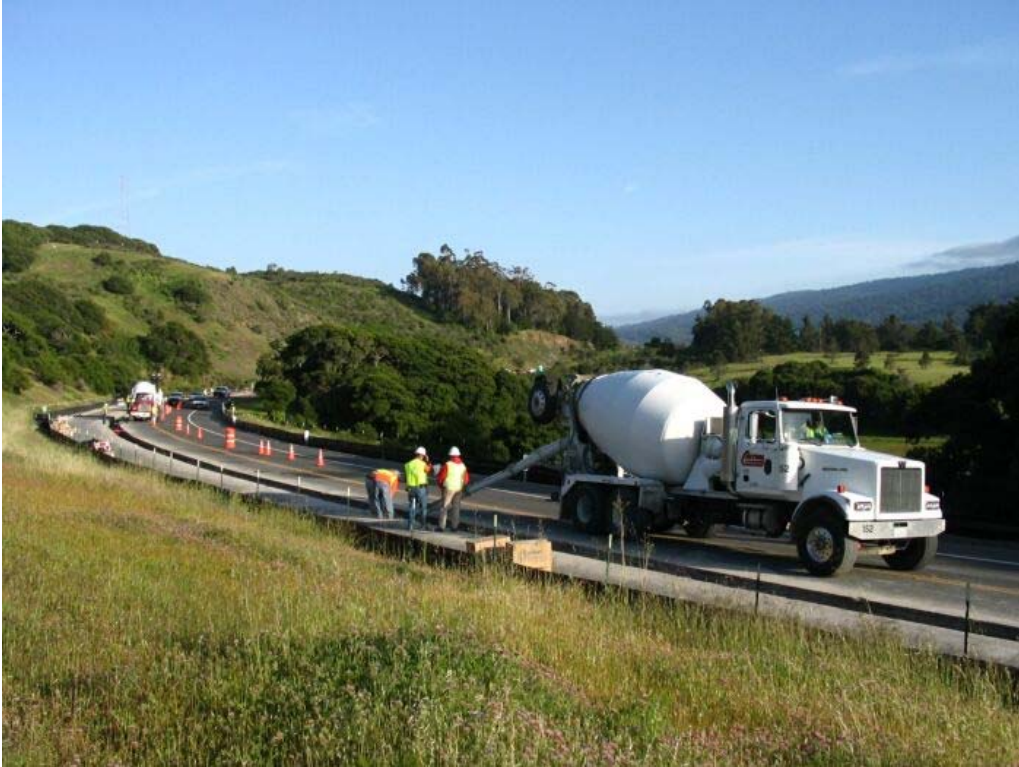
Figure 1 – Crews conducting trenching activities between Manholes #12 and #13 on Cañada Road, Segment 1, April 20, 2005.
