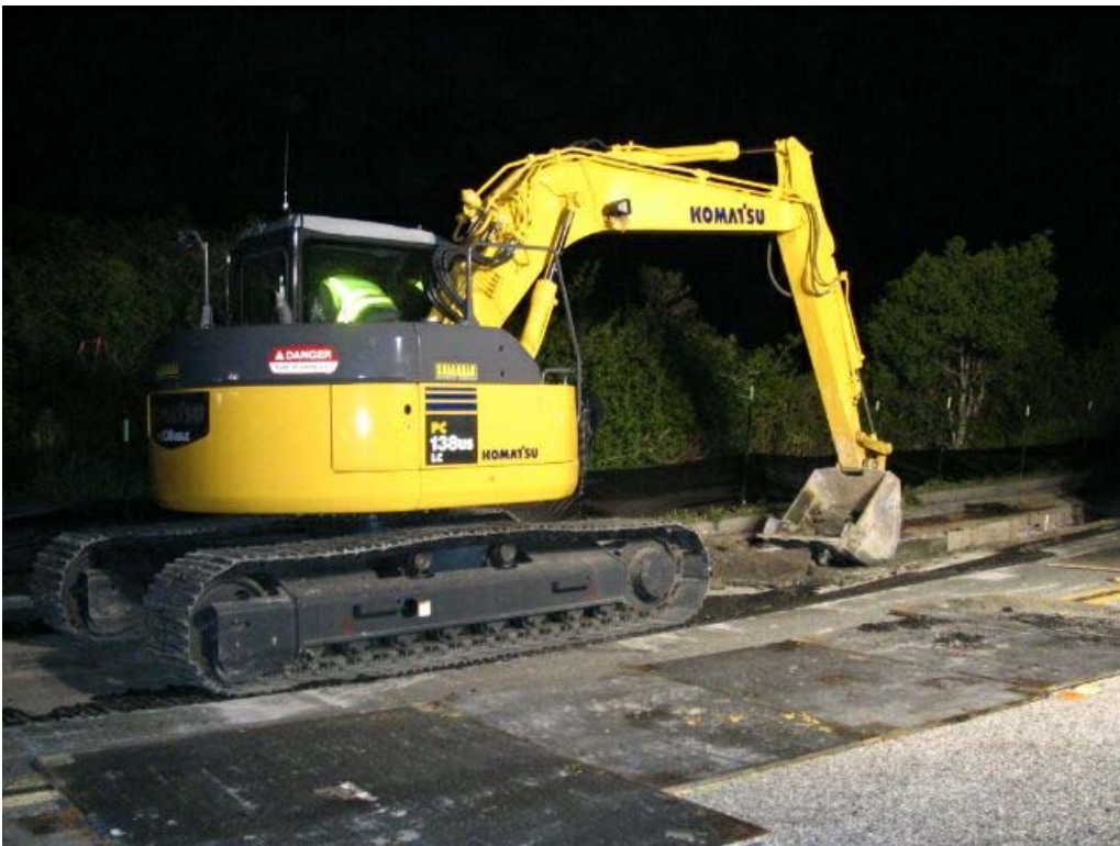
Figure 2 – Crews conducting night trenching activities north of Manhole #20 in the Caltrans area on Skyline Boulevard, Segment 1, April 18, 2005.
