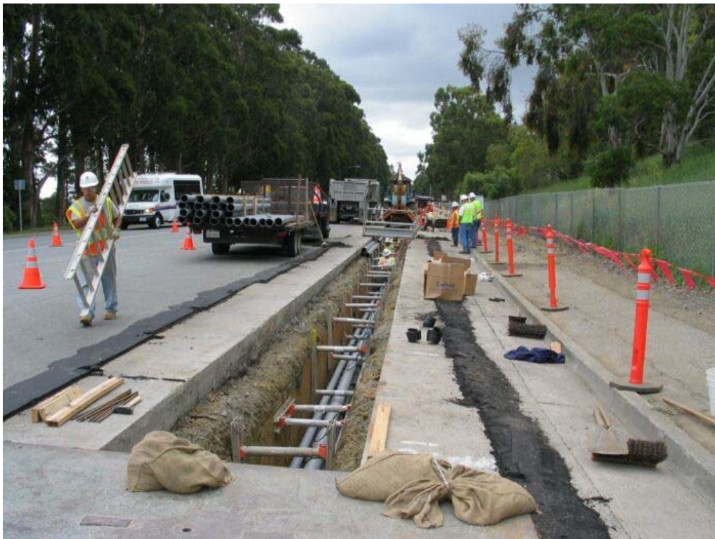
Figure 2 – Crews installing conduit between Manhole #36 and Manhole #37 on Skyline Boulevard, Segment 2 Underground, May 4, 2005.
