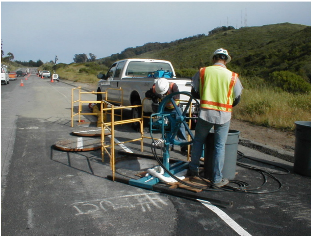
Figure 4 – Crews proofed conduit between Manhole #66 and Manhole #70 on Guadalupe Canyon Parkway, Segment 5, May 4, 2005
