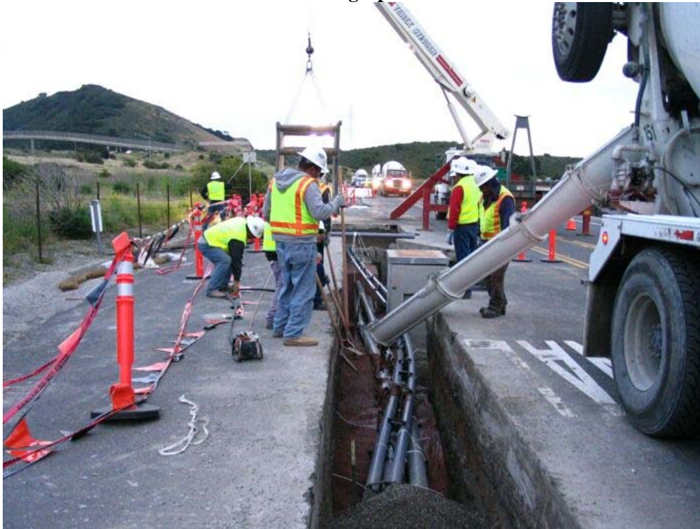
Figure 1 – Crews pouring cement slurry at the Manhole #15 tie-in on north side on Cañada Road, Segment 1, May 3, 2005.
