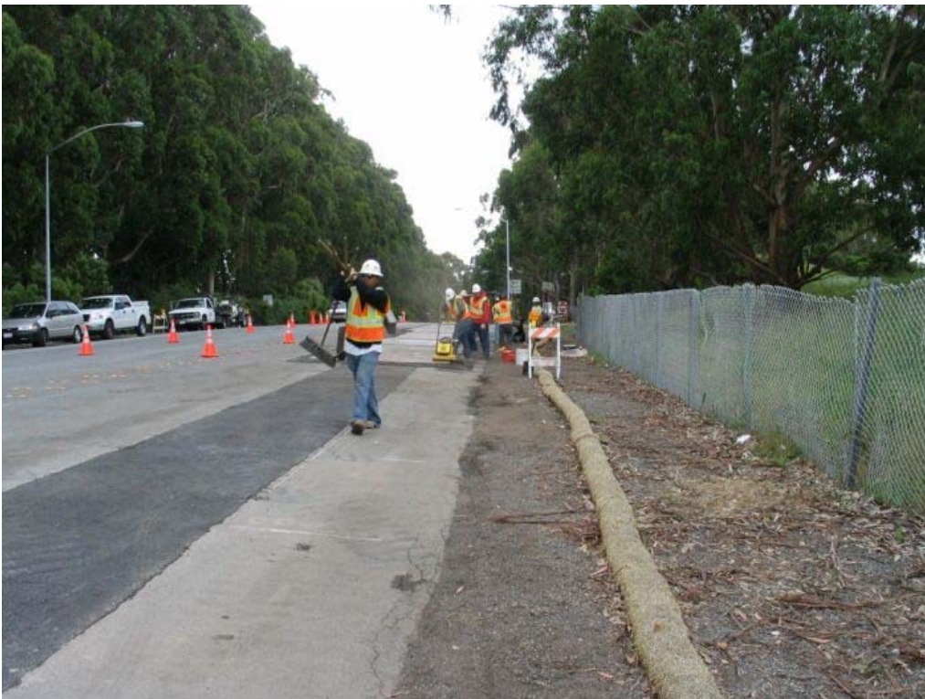
Figure 2 – Trenching area between Manhole #36 and Manhole #37 on Skyline Boulevard, Segment 2 Underground, May 17, 2005
